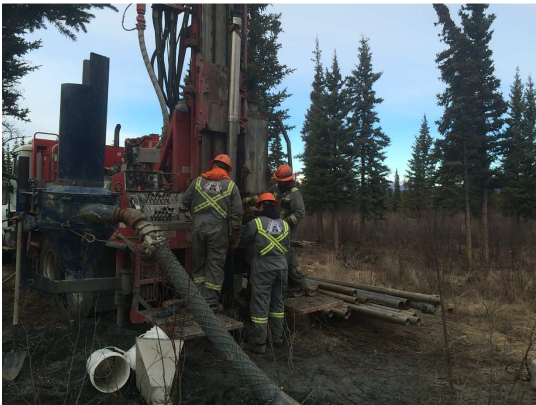
Photo 3: Screen assembly being installed into KFN-M prior to being fitted to the drill string.
