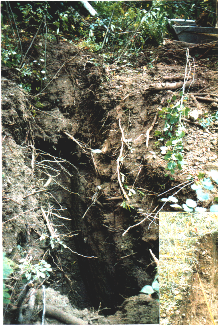
PLATE I5 - Test Pit TPI-7 at north east corner of site between collapsed army buildings.
