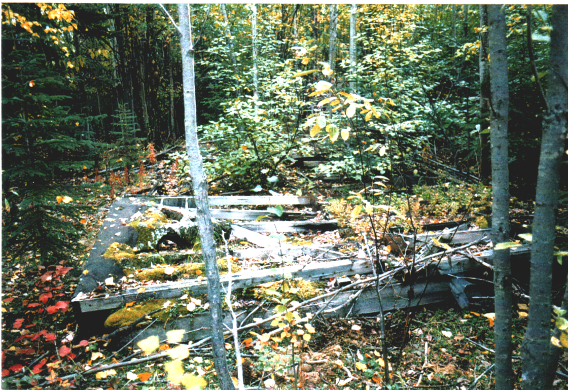
PLATE I2 - One of only two remaining collapsed army construction site buildings.
