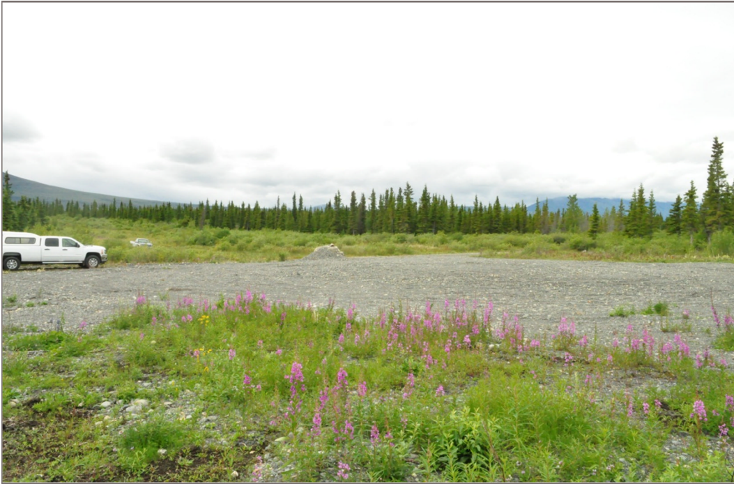
Photo 1: Burwash geoexchange test well drill site prior to arrival of drill. July 16, 2012
