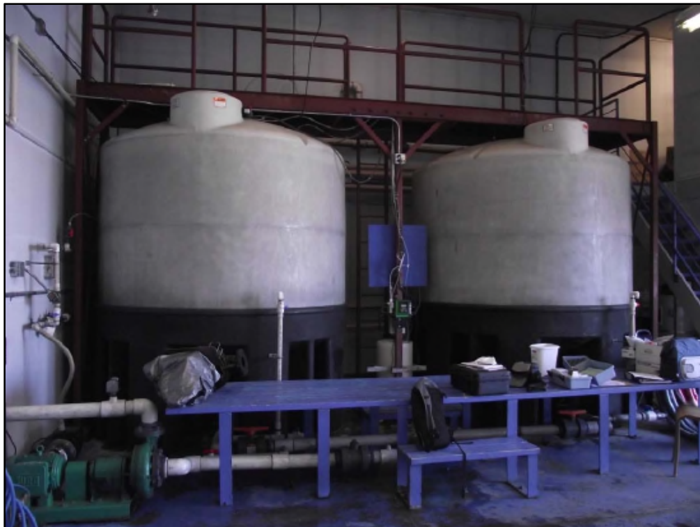
Photo 2: Water Storage Tanks and Fill Pump (July 2011). Note: The building has inadequate space to add additional storage.
