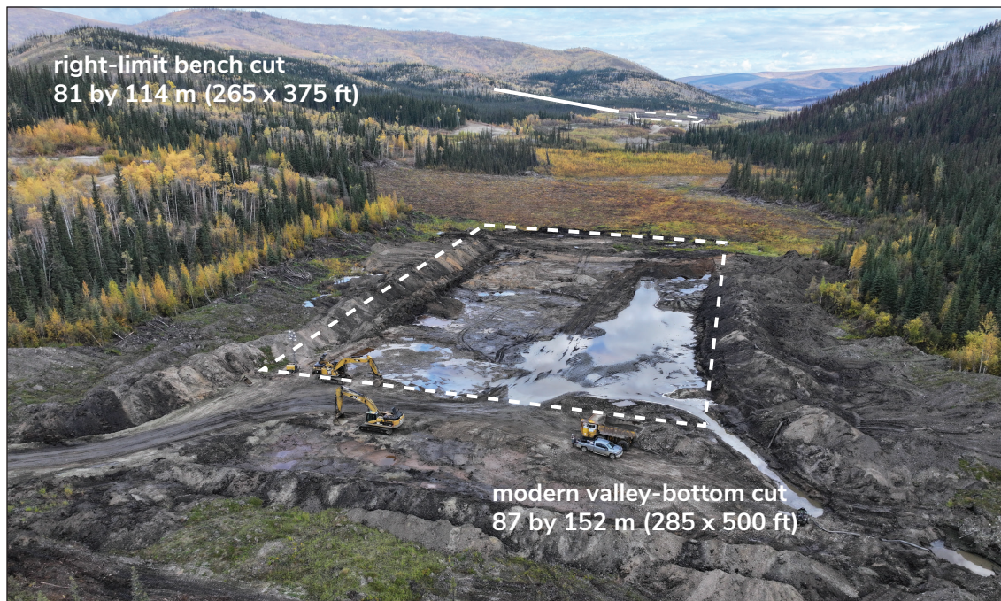
Figure 15. D. Weatherly's two cuts on Black Hills Creek completed in 2025; a right-limit bench cut and a modern, valley-bottom cut. The view is looking upstream.
