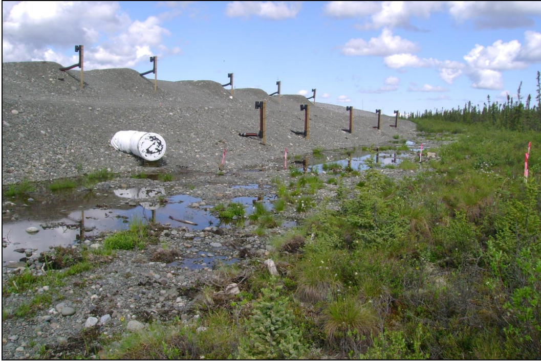
Figure 1. Water ponding on the uphill side of the Alaska Highway embankment, near Beaver Creek, Yukon, Canada. (Photography courtesy of D. Fortier)
