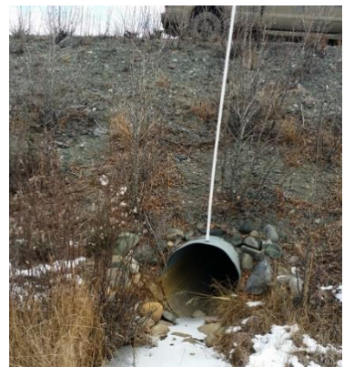
Conditions at outlet to northern 800 mm CSP culvert
