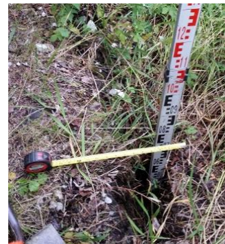
Extension crack along Area # 11
