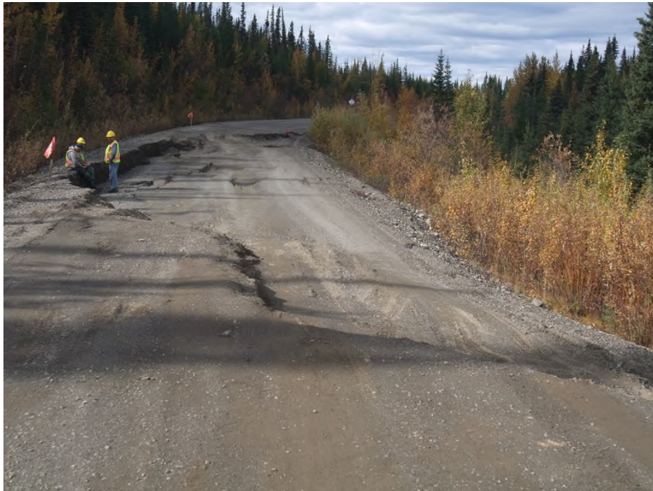
Photo 1: View at km 195 looking north towards Ross River showing slope instability affecting the highway (September 9/15)
