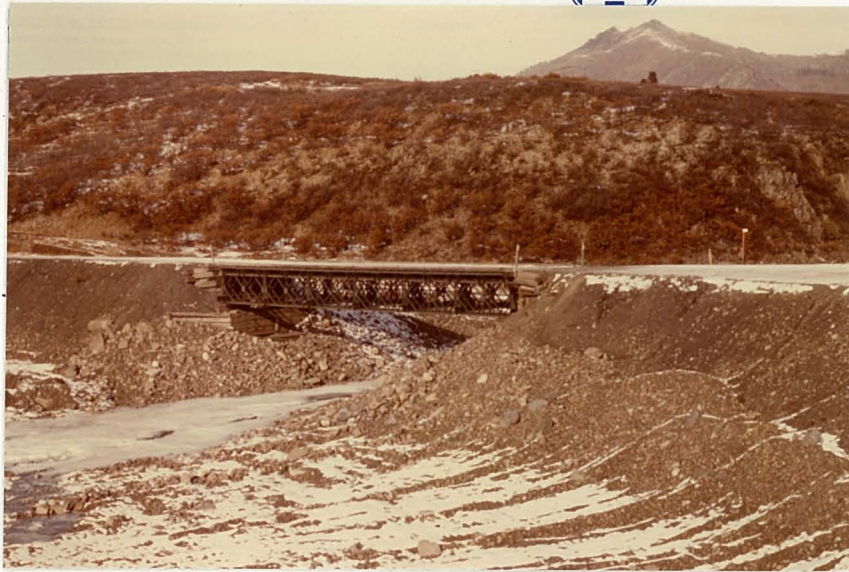
Photograph No. 11: The existing Bailey Bridge over the Upper North Klondike River at approximately Mile 47.8. Upstream is to the right of the photograph.
