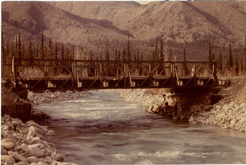
Photograph No. 7: The existing Bailey Bridge at Wolf Creek at approximately Mile 31.4, looking upstream. This Bailey Bridge has a 40 foot span and is of single-single construction. It is to be replaced with a steel beam bridge. Note the abundance of coarse granular material in the stream bed and the proximity to the mountains in the background.
