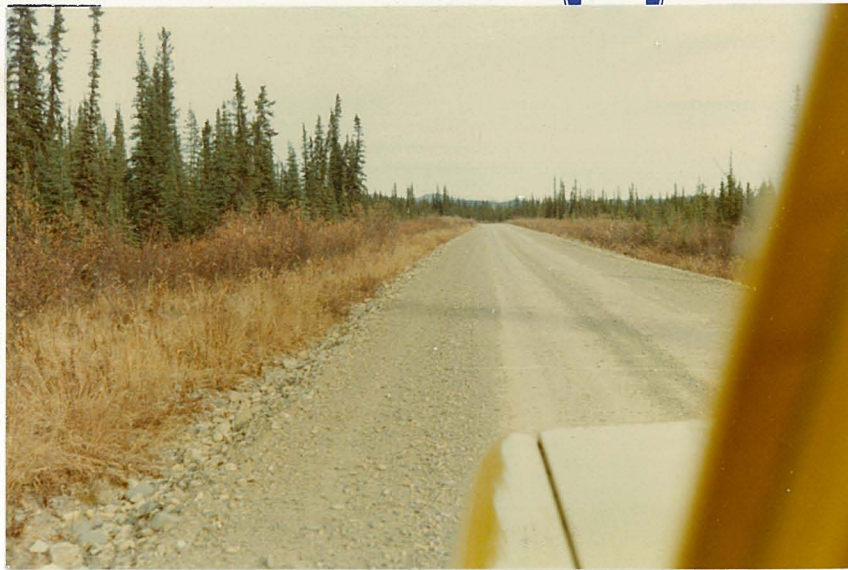
Photograph No. 3: A view of the existing grade at approximately Mile 5 looking north. Note the excellent state of this section of the highway which is typical of long stretches between Mile 0 and Mile 60. The tree cover on the left is typical for the first 43 miles of the highway. The dominant tree is white spruce.
