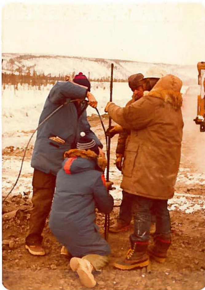
8. The installation of the monitoring system by NRC. The thermistor cables reach to a depth of about eleven (11) feet with thermistors at one to two foot intervals.
