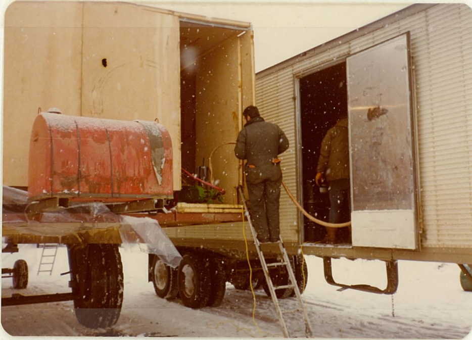
13. Pumping the foam producing liquids from 45 gallon drums to the machine. The liquids were not warm and so presented difficulty pumping.
