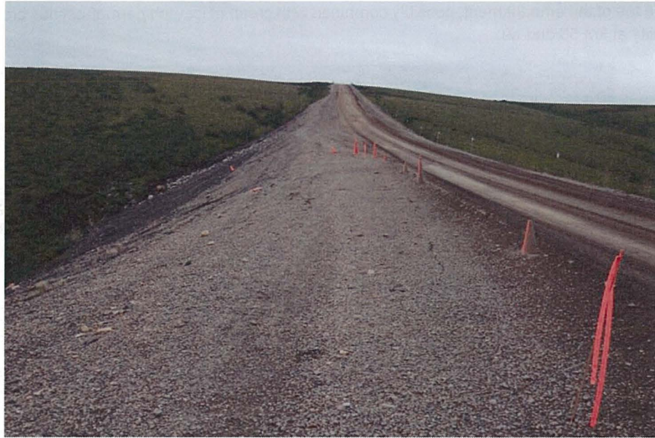
Photo 17: Road instability related to tension cracks and slumping on a deep fill at km 30 NT (August 25, 2013)
