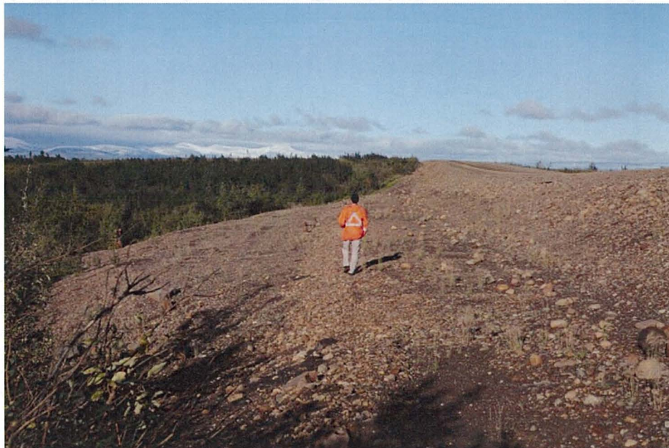
Photo 18: Successful application of a toe berm to stabilize road embankment km 51 NT (August 25, 2013)
