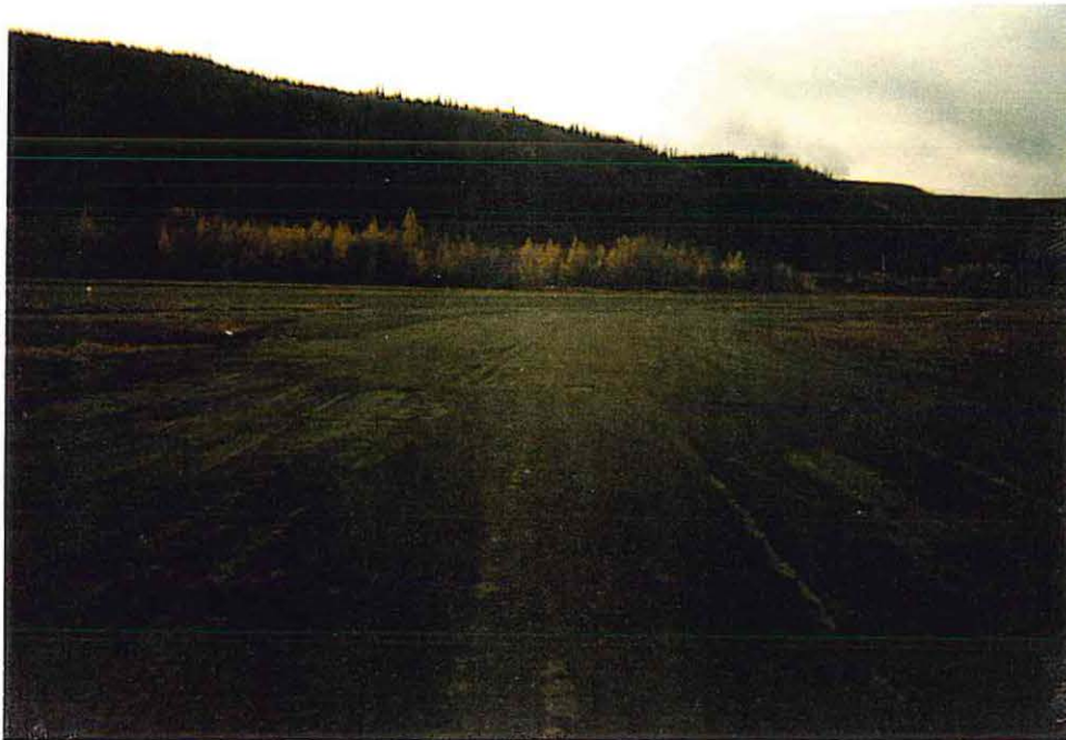
PHOTO # 9 – Repair Area 1 – Final Grade – Note the runway location in the background.
