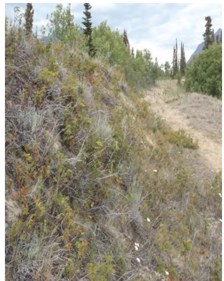
Showing how cut slopes with dense vegetation can be constructed with steeper slopes
