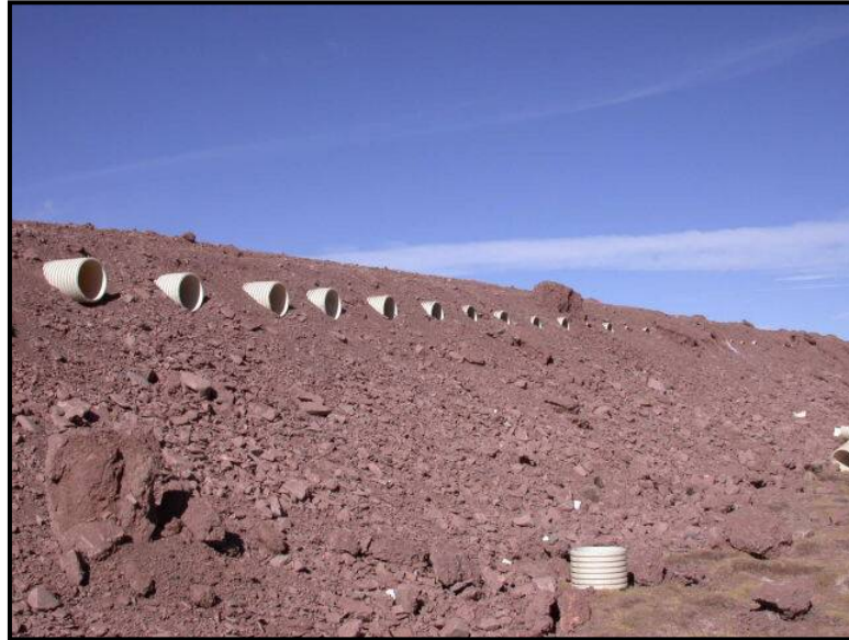
Figure 2-12: Ventilated embankment with cuverts, Qinghai-Tibet Roadway, Tibetan Plateau (Courtesy of Professor Ma, Lanzhou, China)
