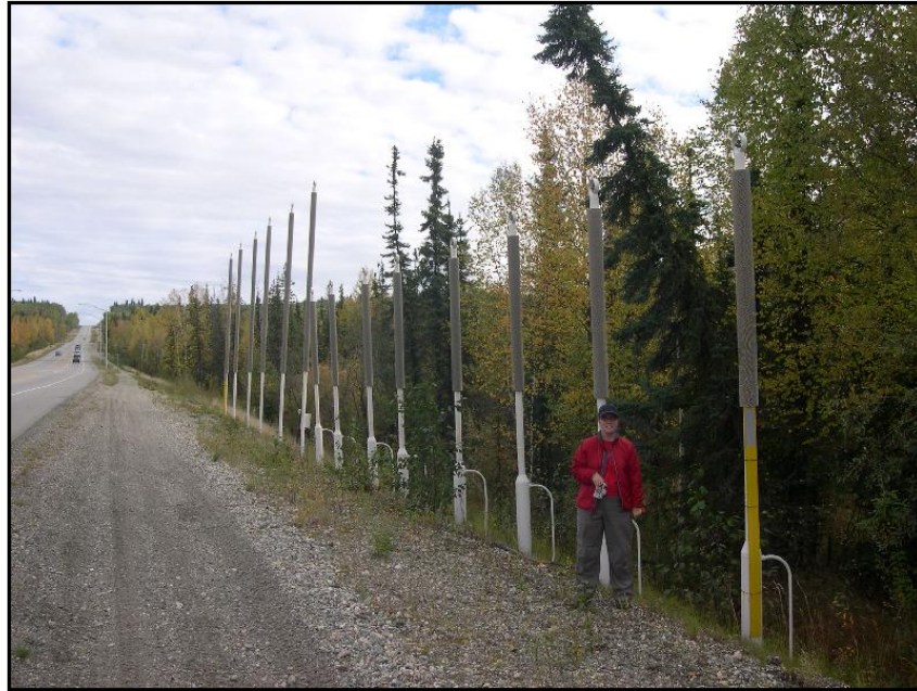
Figure 2-13: Horizontal thermosyphons on Chena Hot Springs Road, Alaska
