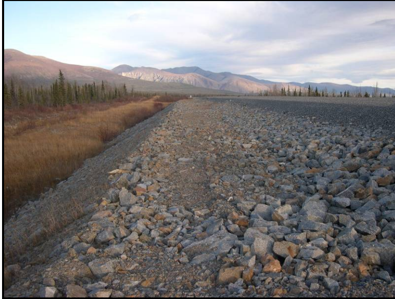
Figure 2-20: Rock Berm on Alaska Highway, Yukon, Canada (Photo by Guy Doré, Université Laval)
