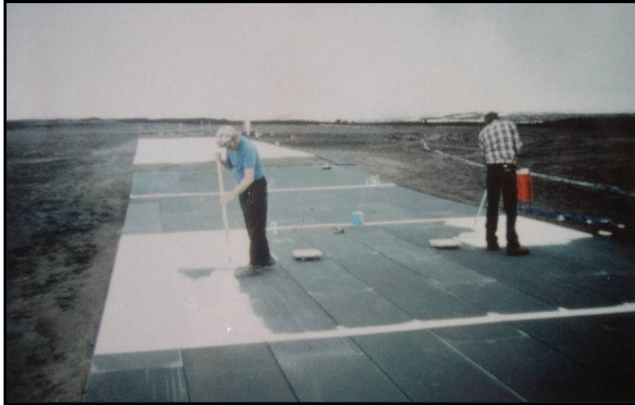
Figure 2-9: Workmen applying white paint on a test section (courtesy of Cold Region Research and Engineering Lab, CREEL)
