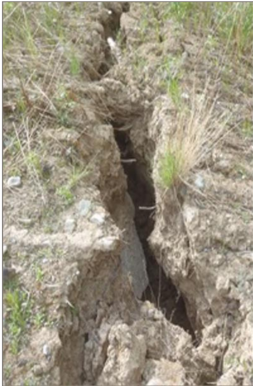
Photo 3: Longitudinal cracking in embankment atBH01, June 18, 2013
