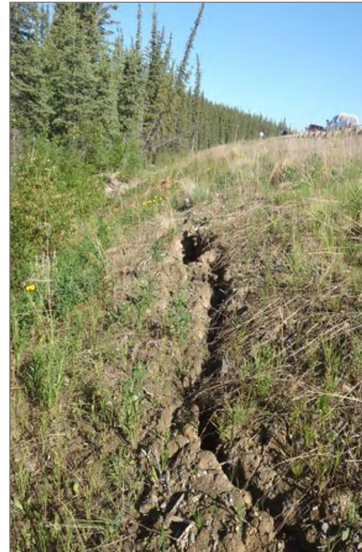
Photo 4: Longitudinal cracking along south bound embankment, aspect NW, June 18, 2013
