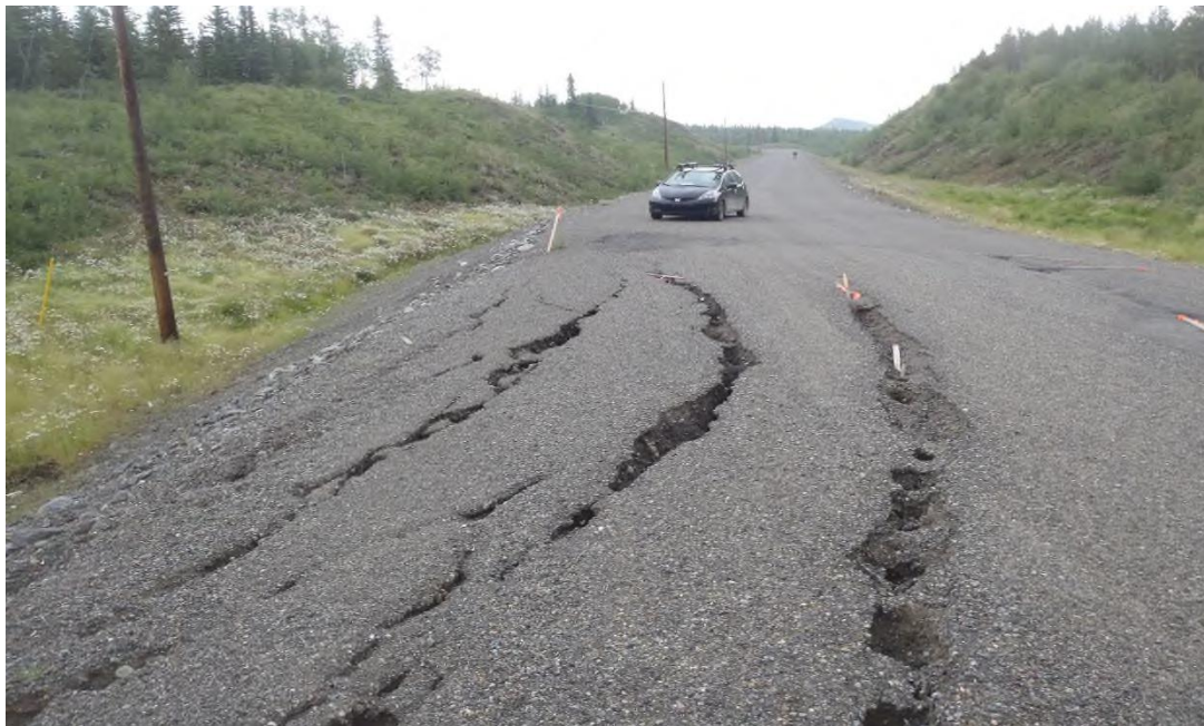
Photo 1: July 9, 2015 - Subgrade Failure at Sta 6+670
