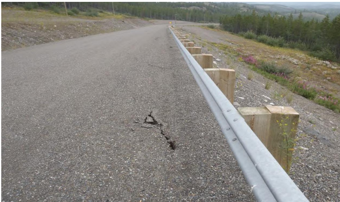
Photo 3: July 9, 2015 – RHS Embankment Instability North Of Sta 6+100
