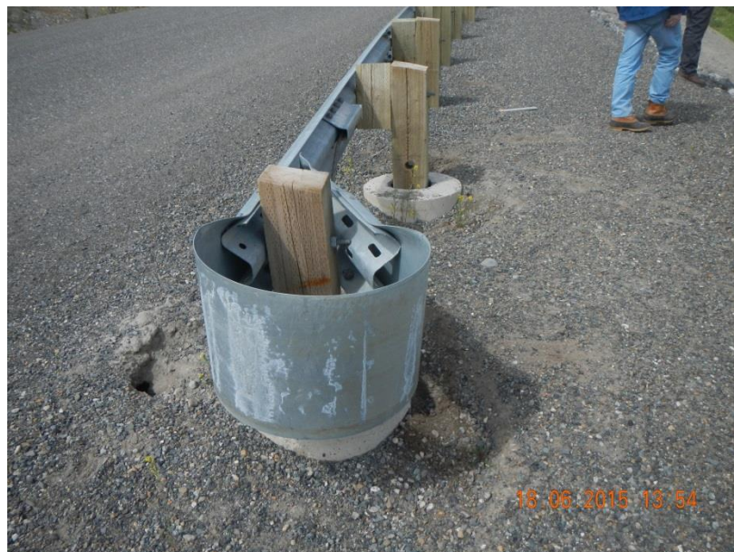
Picture 3-10 Erosion around concrete guiderail abutments.
