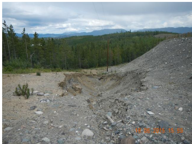
Figure 3-6 Major scour in ditch around 6+400 on the left hand side.
