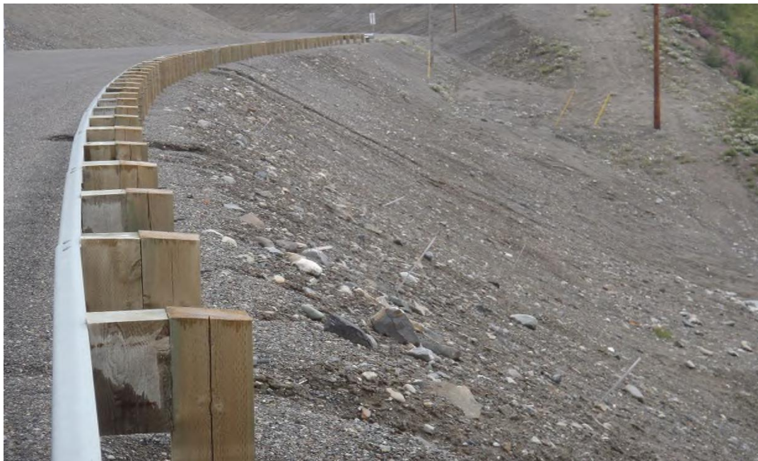
Photo 5: July 9, 2015 – Sta 5+280 RHS – Wash-outs Along Guard Rail
