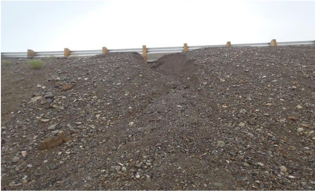
Photo 6: July 9, 2015 – Sta 2+060 to Sta 2+300 – RHS – Washouts Extending Under Guardrail & Barrier Curb
