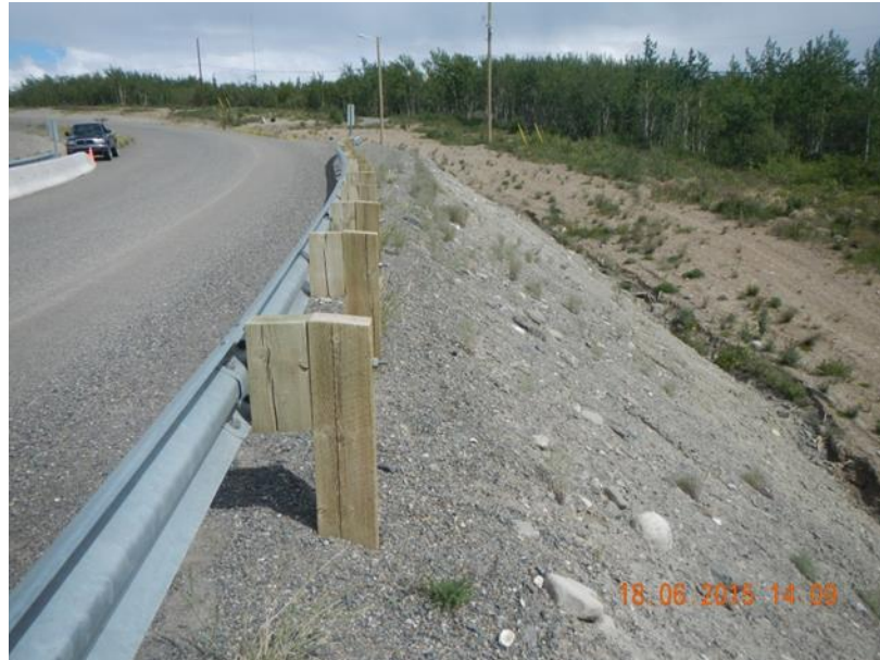
Figure 3-9 Guiderail installed in the embankment slope at 2+100 on the left hand side. Also note the scouring in the ditch bottom.
