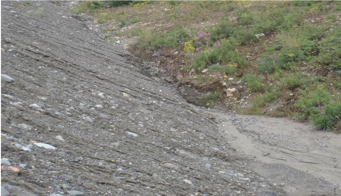
Photo 2: July 9, 2015 – Ditch Scour at Sta 6+320 (greater than 3 m at some locations)
