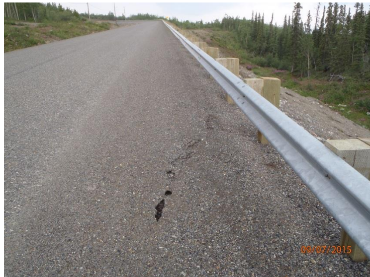
Picture 3-1 Tension cracking extending up the fill embankment and into the BST surface at 0+850 on the right hand side.
