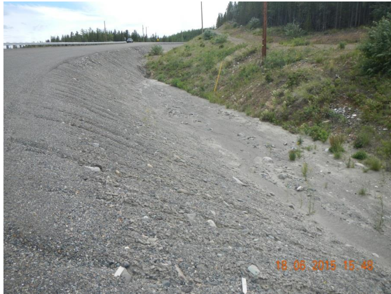
Picture 3-8 Deposition of fine grained material in the ditch bottom has plugged the culvert inlet at 6+050 on the LHS.
