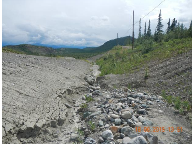
Picture 3-5 Ditch scour and downstream deposition around 0+800 on the left hand side.
