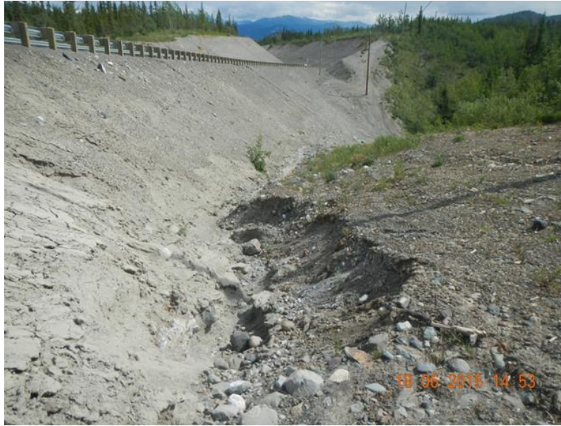
Picture 3-7 Major scouring located in a transition from cut to fill on the right hand side of road 5+140.
