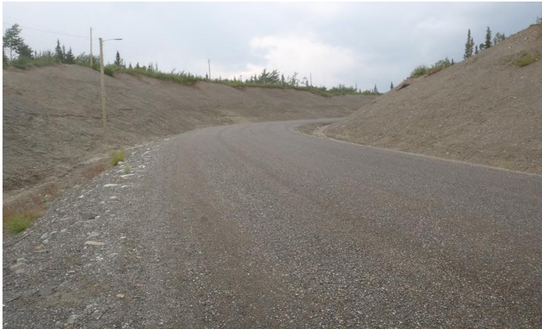
Photo 4: July 9, 2015 – Surficial Erosion Along High Backslopes at Sta 5+550 – Ditches Carrying Sediment
