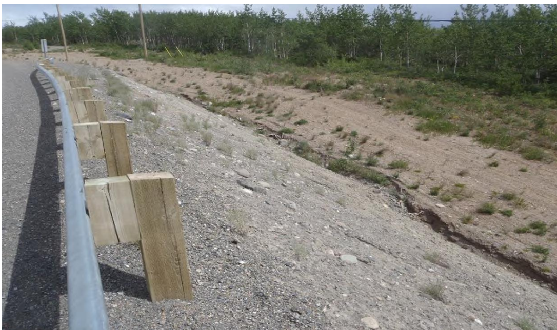
Photo 7: June 18, 2015 – Sta 2+150 – LHS – Ditch Line Scour Down-gradient of Transition to Large Fill Area
