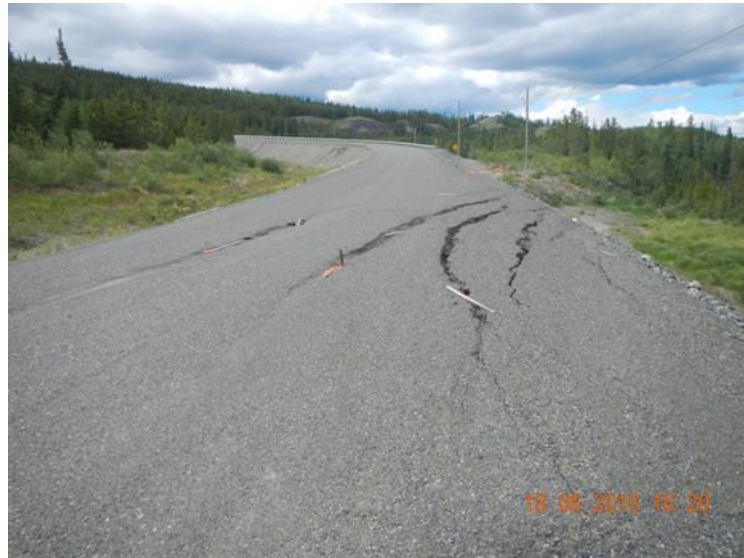
Picture 3-2 Localized failure of the road subgrade at 6+670.
