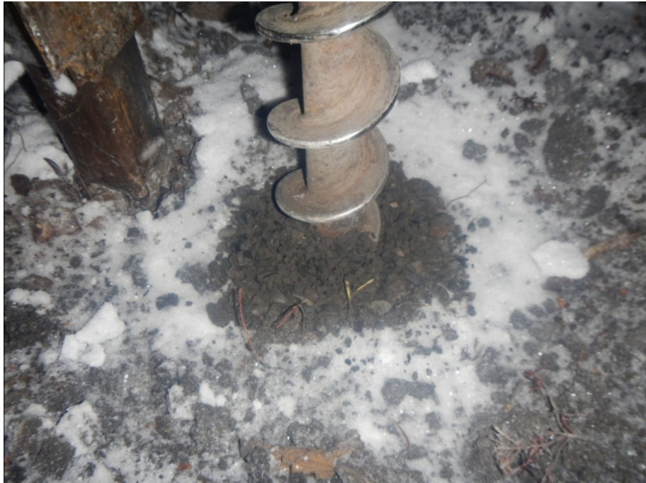
Figure 905-6607.1 Photo of auger cuttings from borehole 905-6607 representative of soil strata between 2.4 and 3.7m
