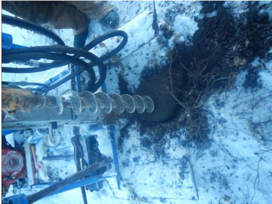
Figure 905-6596.2 Photo of drill cuttings coming up auger in borehole 904-6595 from 0.4 and 1.0m
