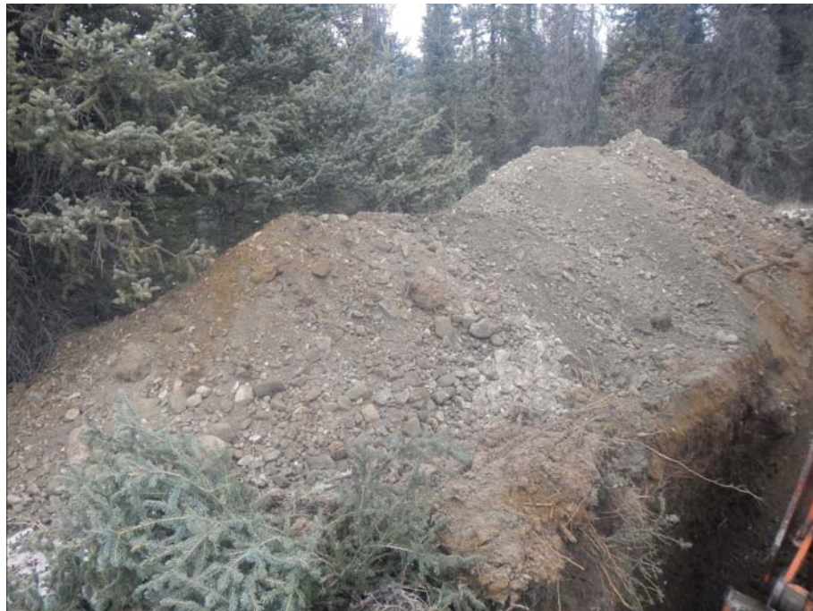
Figure 906-6562.2 Photo of waste piles from test pit 906-6562
