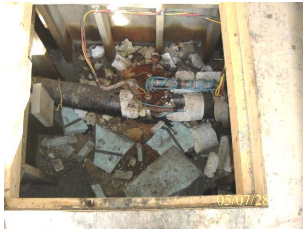
Photo 0594: 3957 Wellhead in pit below floor at well house
