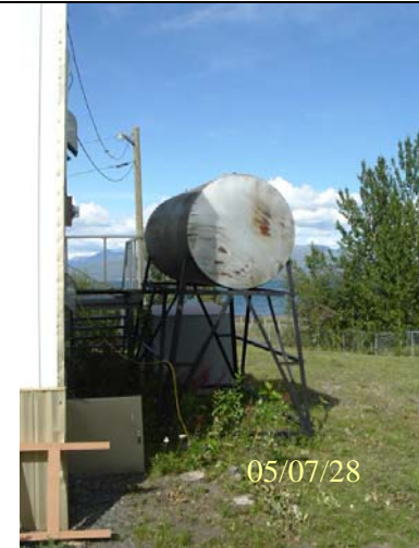
Photo 0591: 3957 Above ground fuel storage tank
