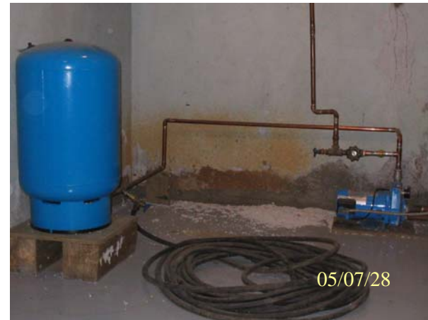
Photo 0114: 3201 Pressure tank (left), and jet pump (right)
