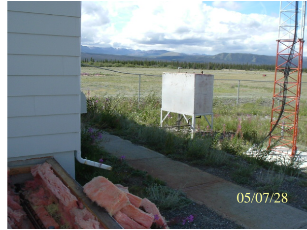
Photo 0579: 3201 Above ground fuel storage tank
