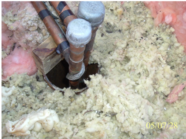
Photo 0577: 3201 Wellhead. Note open casing.
