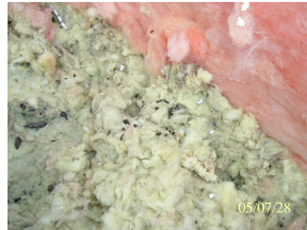
Photo 0578: 3201 Insulation around wellhead with evidence of mouse feces
