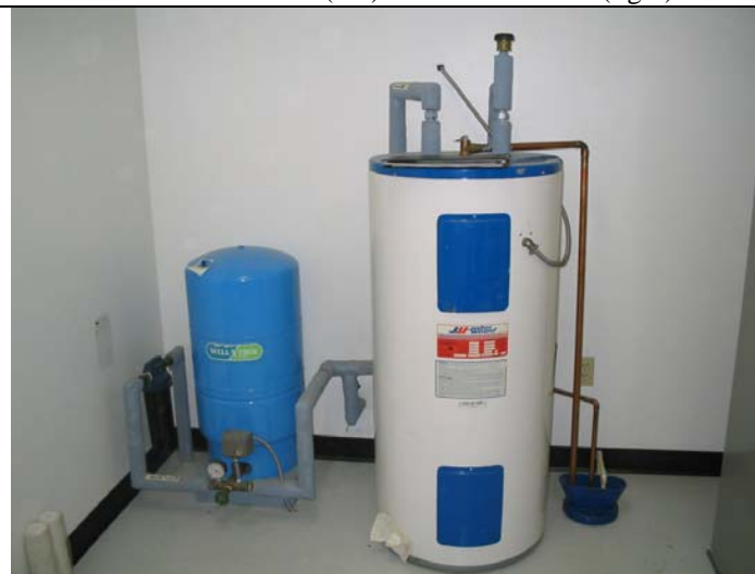
Photo 0018: 6522 Pressure Tank (left) and Water Heater (right)
