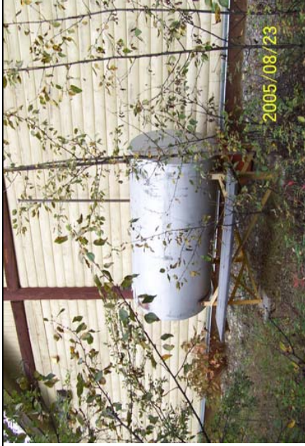
Photo 403: 5678 On site AST on west side of building.
