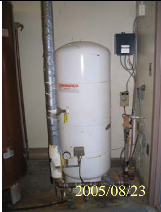
Photo 208: 5672 Water system. (pump controls, pressure tank)
