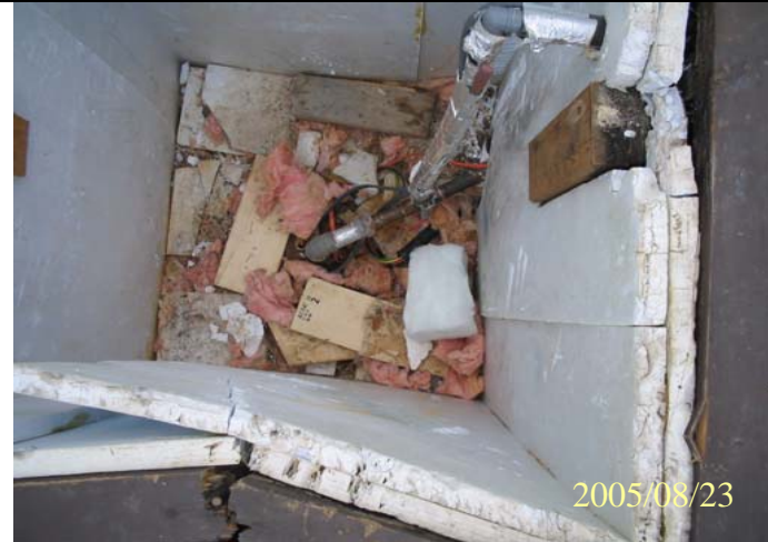
Photo 209: 5672 Well enclosure and wellhead.
