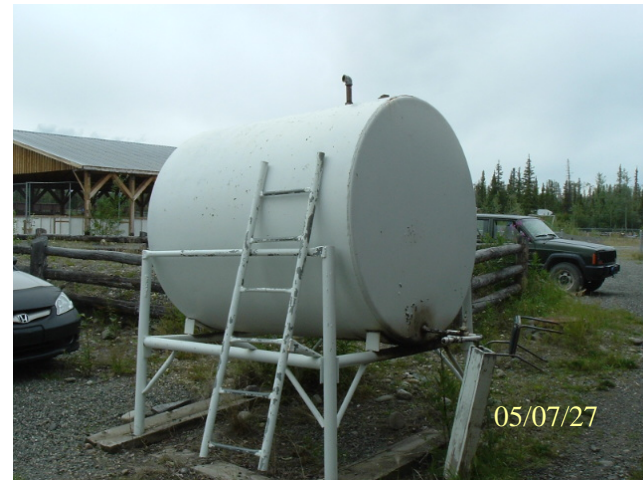
Photo 0539: 3122 Above ground fuel storage tank
