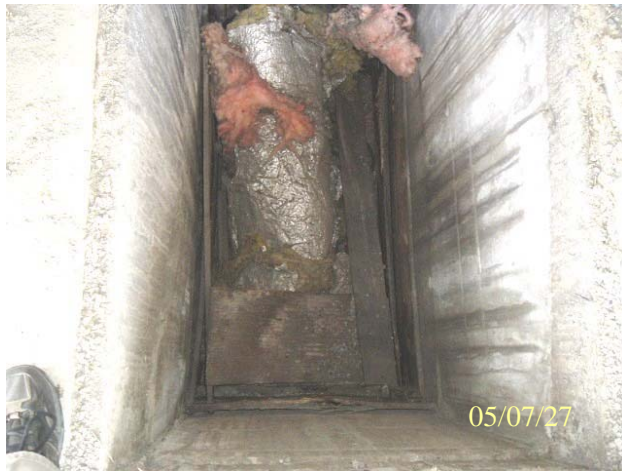
Photo 0535: 3122 Wellhead in pit
