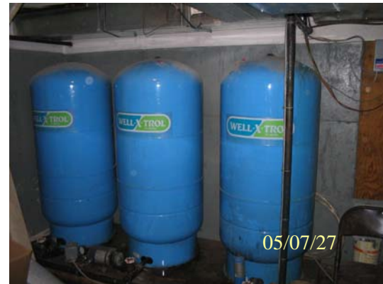
Photo 0087: 3122 Pressure tanks in crawl space of Community Club
