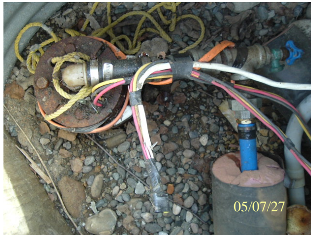
Photo 0561: 3121 Wellhead in pit
