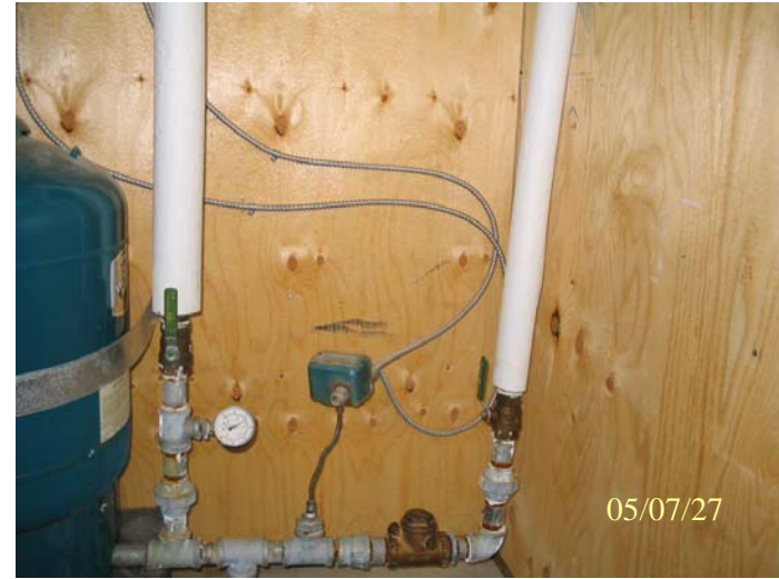
Photo 0099: 3121 Point of entry and pressure tank
