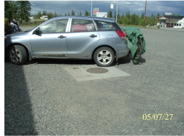
Photo 0559: 3121 Wellhead enclosure in parking lot
