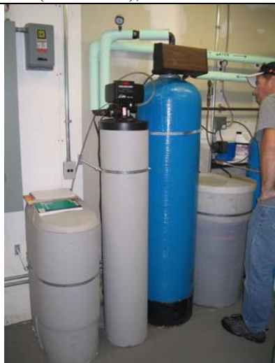
Photo 0026: 4951 Water softener (left), greensand filter (centre), and brine tank (right)
