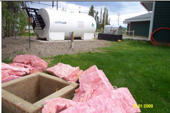
Photo 0217: 4951 Wellhead enclosure (front), doubled walled enviro tank above ground fuel storage tank (back left), existing above ground storage tank with secondary containment tub (back centre), and Teslin Health Centre (back right).
