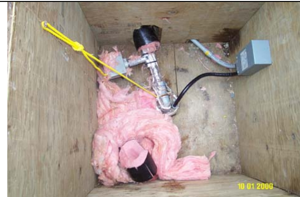
Photo 0216: 4951 Wellhead in pit
