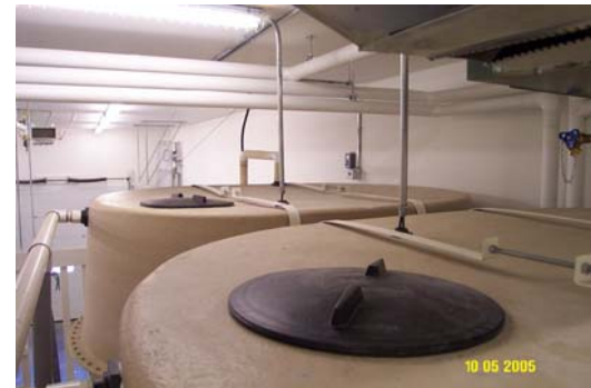
Photo 0097: 1421 Water Storage Tanks (in firehall)
