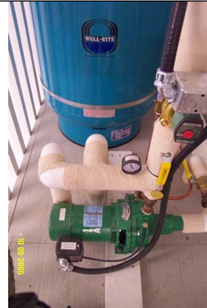
Photo 0098: 1421 Pressure Tank and System
