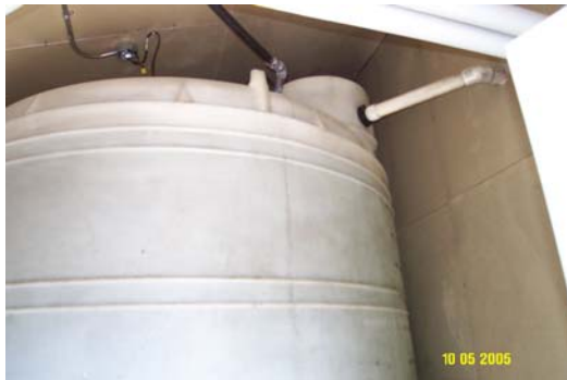
Photo 0088: 1421 Water Reservoir (in wellhouse)
