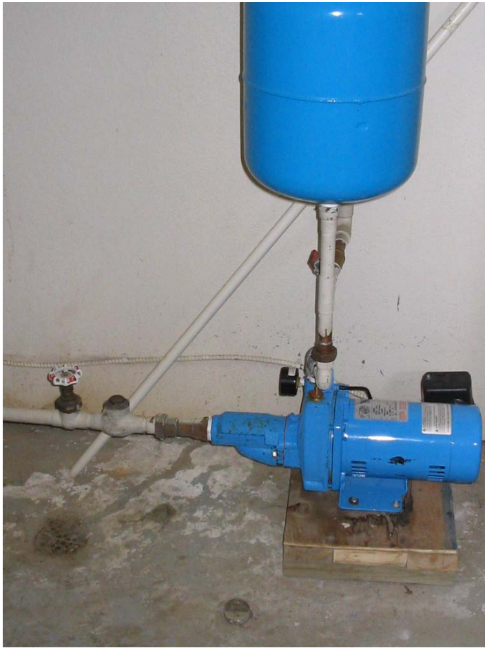
Photo 0059: 6746 Jet pump and pressure tank
