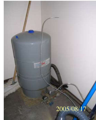
Photo 0189: 5653 Pressure tank and pump controls.
