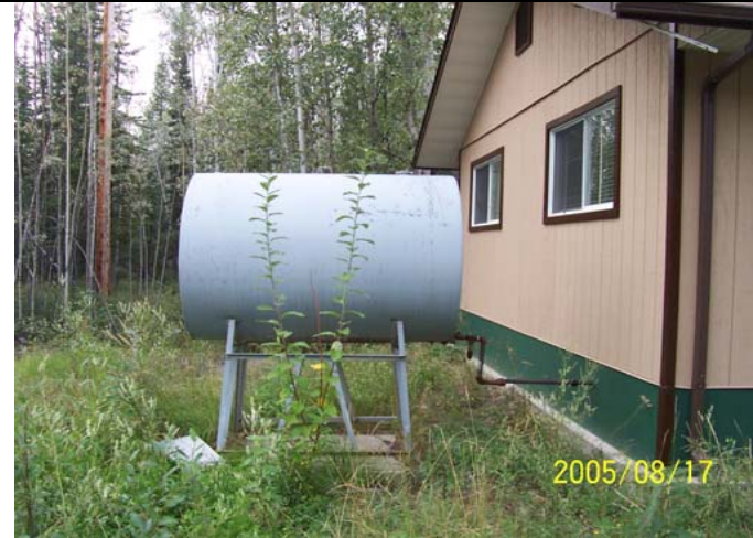
Photo 057: 5650 On site AST.
