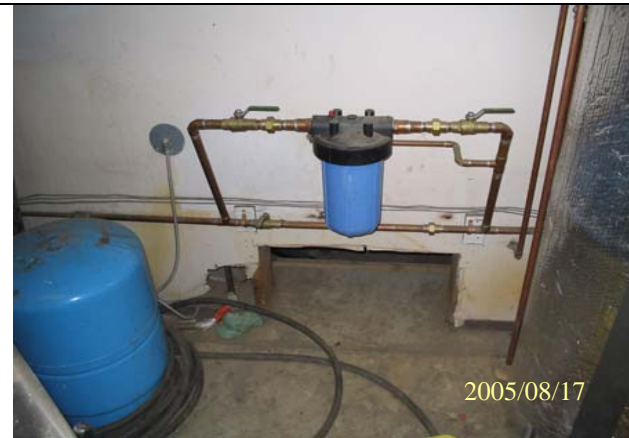
Photo 194: 5650 Water system. (pressure tank and filter)
