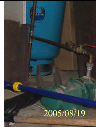
Photo 237: 2592 Jet pump and pressure tank.
