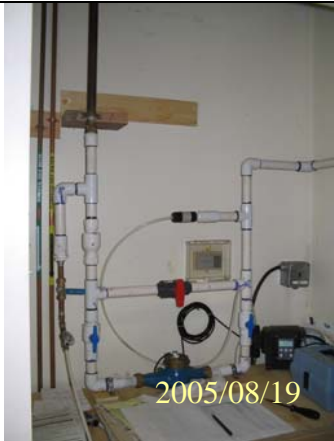
Photo 236: 2592 Chlorination system, flow meter, and associated plumbing.
