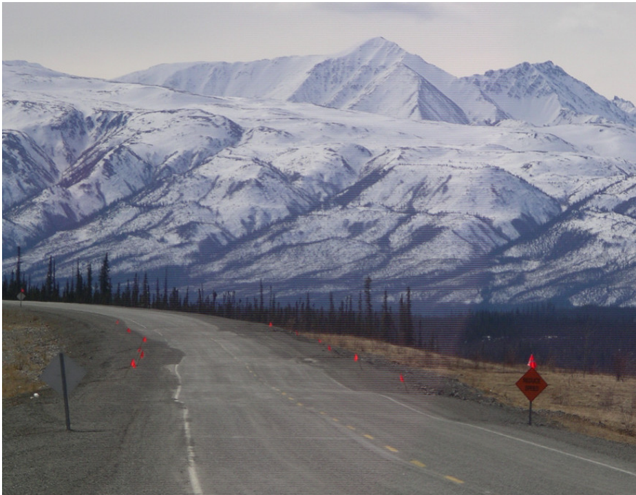
Figure 6 Subsidence along the Alaska Highway due to permafrost degradation, 50 km south of Beaver Creek.
