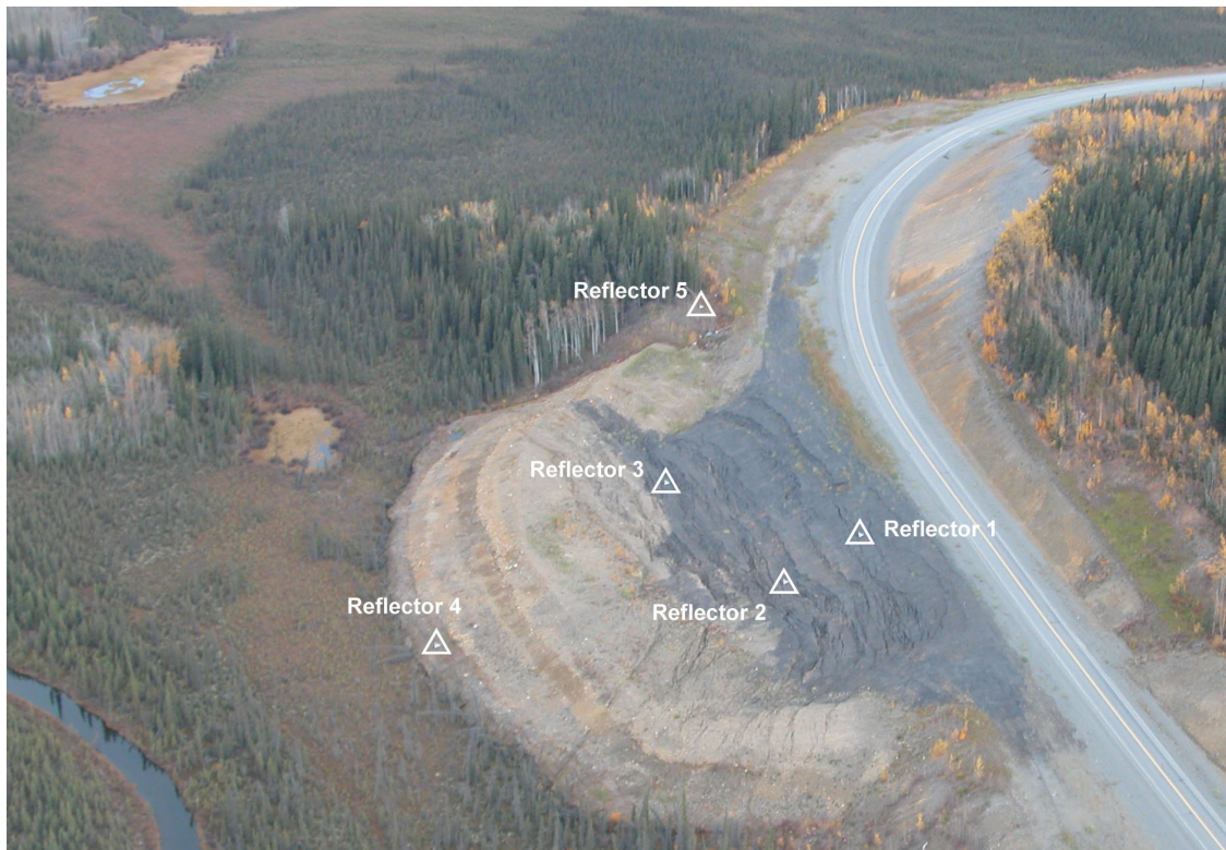
Figure 7 Embankment failure due to permafrost degradation at Beaver Creek, Site 1, along the Alaska Highway.
