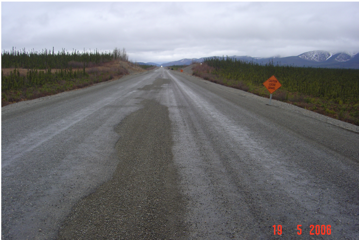
Figure 9 Patched cracks in the road are evidence of thaw settlement along the Alaska Highway at Beaver Creek, Site 2.
