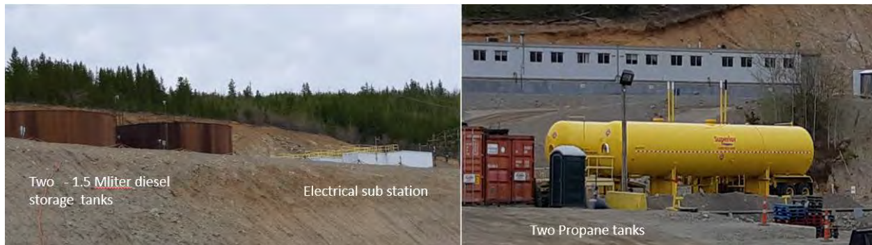
Figure 18-4: Substation and Fuel Storage
