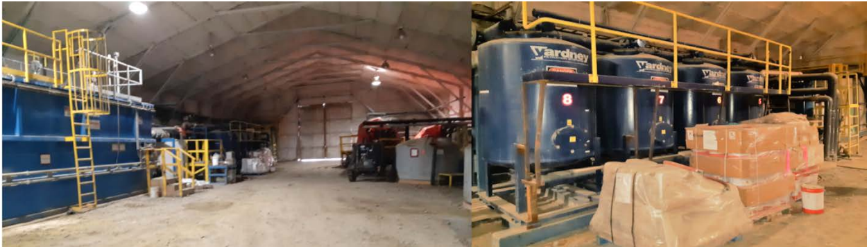
Figure 18-7: Reverse Osmosis Plants for Water Treatment
