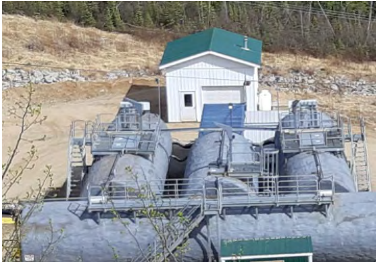
Figure 18-6: Sewage Treatment Plant
