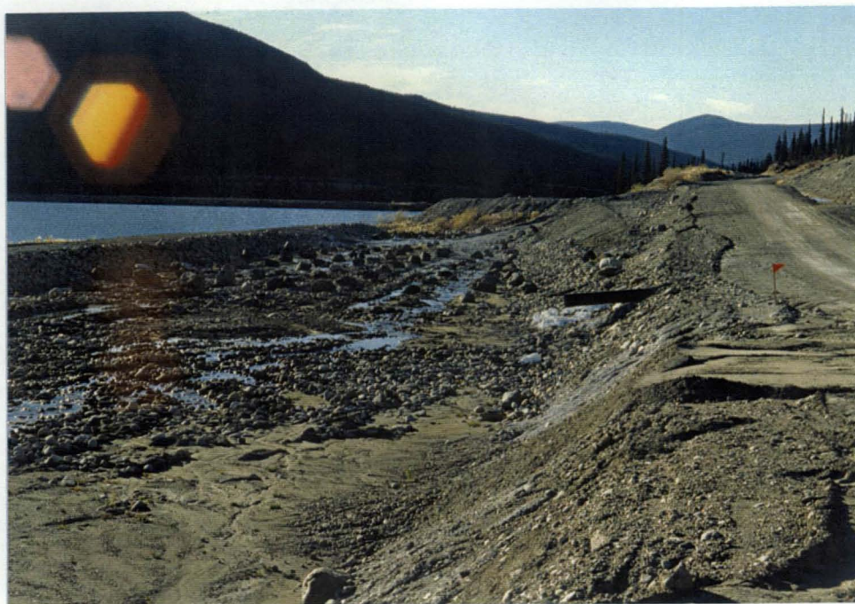
The upper photo is a general view of the gently graded spillway section with the retaining dyke to the left. The lower photo, taken from the dam crest, illustrates the crest of the spillway dyke. The dyke needs to be raised further, in spite of work done in late 1994.
