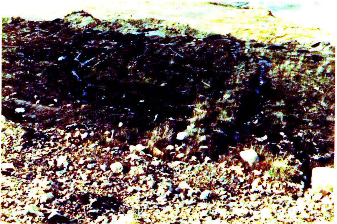
Photo 8 Evidence of seepage from diversion ditch
