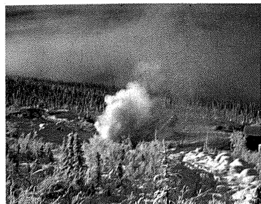
The first round being blown at the portal site, to start the underground program.
