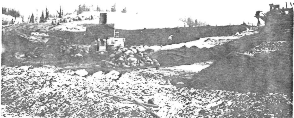
PLATE 12: Oct. 3/90. Covering finger drains "T1" and "T2" with filter fabric and constructing the rock drain at the end of "T1."
