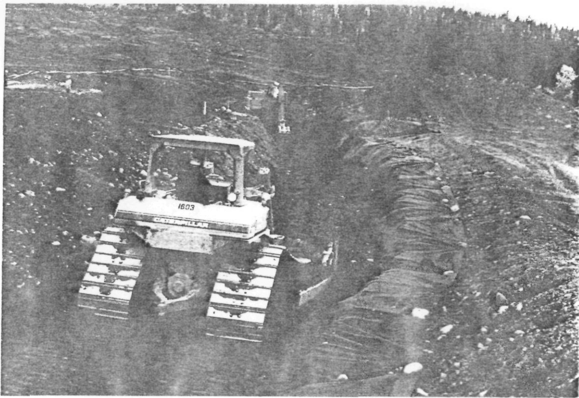
PLATE 5: Sept. 14/90. The cutoff trench is then backfilled in thin lifts which are placed initially by the backhoe and then tracked down with a dozer in preparation for compaction.
