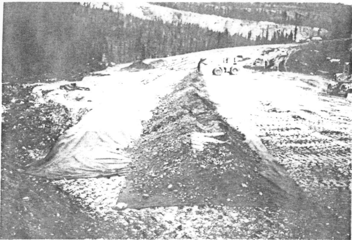
PLATE 11: Oct. 1/90. View northwards from Sta. 0+040 at the construction of finger drain "L1."
