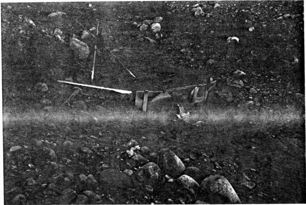
Photo 16: Heavy seepage from the north abutment.
