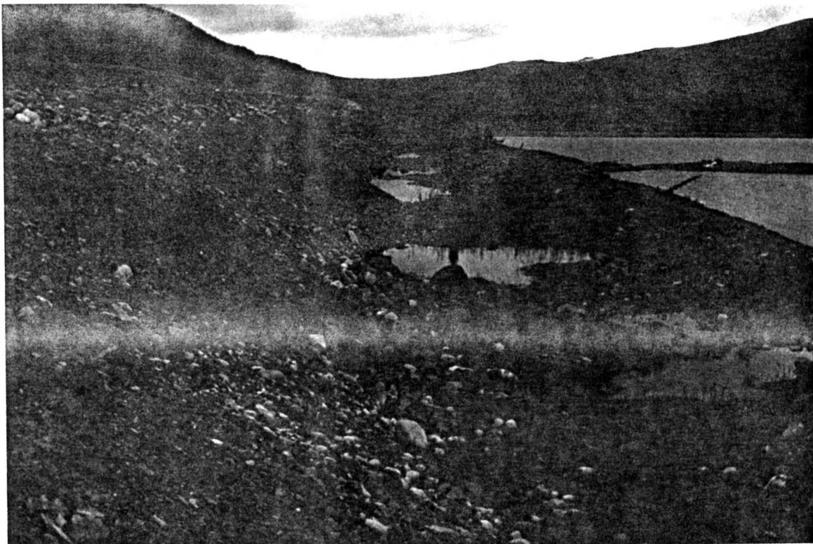
Photo 9: Seepage from the canal is ponded in localized depressions along the toe of the dyke.
