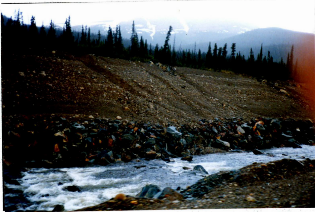
Photo 9 - Cut slope erosion above Rose Creek diversion. If the erosion becomes excessive these channels should be filled with small waste rock.
