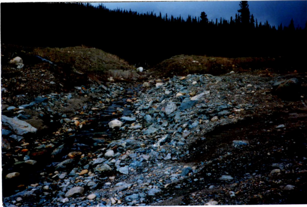
Photo 1 - N.W. interception trench. Limited scour has taken place. Some maintenance desirable to upgrade ditch to carry flood flow.
