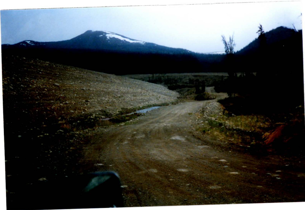
Photo 6 - Downslope area of Cross Valley dam. Note seepage at left.
