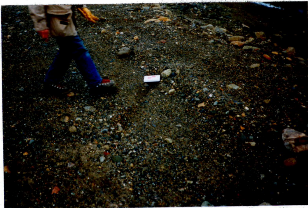
Photo 10 - Crack across the Rose Creek diversion dyke. This slope has moved toward the tailings pond. The slope should be stabilized. Horizontal drains are a low cost stabilization procedure.
