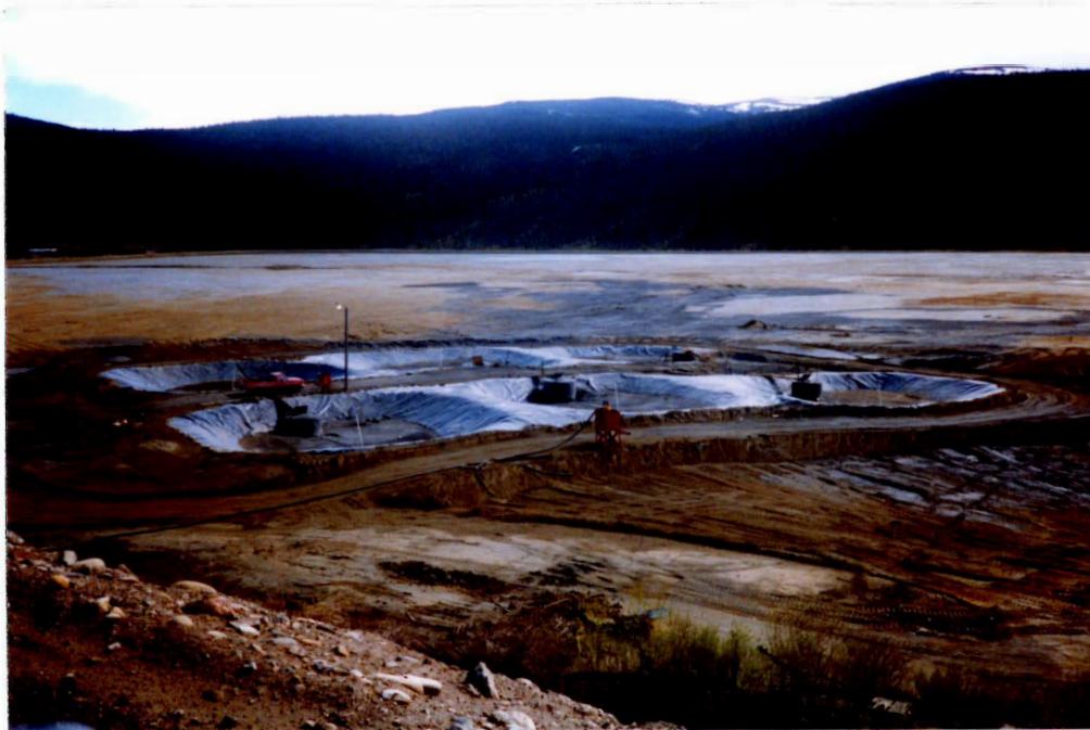
Photo 19 - Test plots in the old tailings pond to evaluate acid generation under various conditions.
