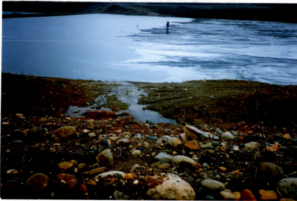
Photo 11 - Seepage through the Rose Creek diversion dyke. Some piping is also occurring. A sandy gravel filter cover and horizontal drains are recommended.
