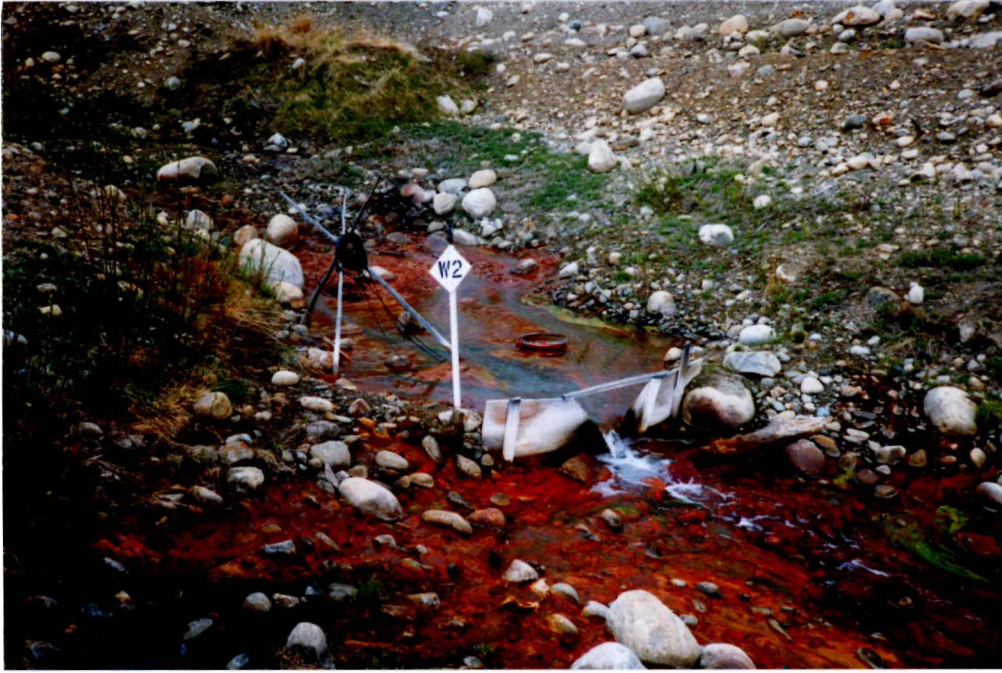
Photo 5 - Seepage exiting below the north end of the Cross Valley dam. A V notch gauge installed to measure seepage. W2 is a water sampling station for metals and chemical analysis. The volume of seepage is considerable. The water must be monitored closely to evaluate if any piping (loss of soil) is occurring. If it is a collection pipe and granular toe term are recommended.
