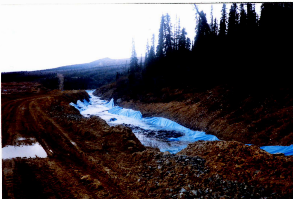
Photo 20 - Diversion of N. Fork around the open pit. Plastic lining has been placed to reduce seepage and pumping from the pit. This is a temporary program until the pit is mined out and the water will likely be diverted into and through the pit.
