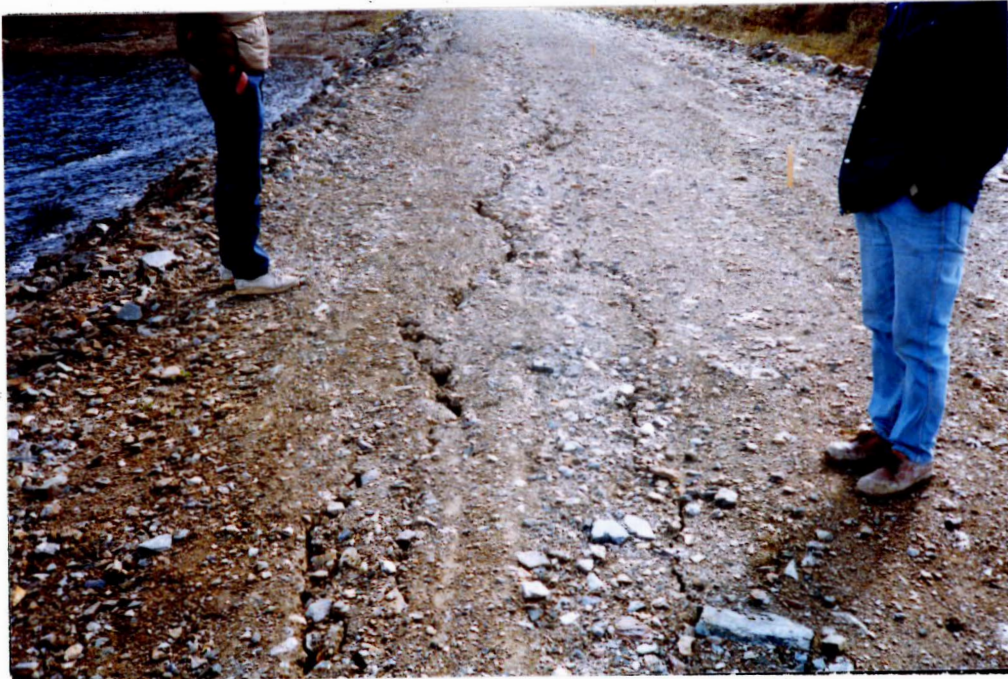
Photo 17 - Crack on top of fresh water dam. The cause must be definitely determined and corrected.
