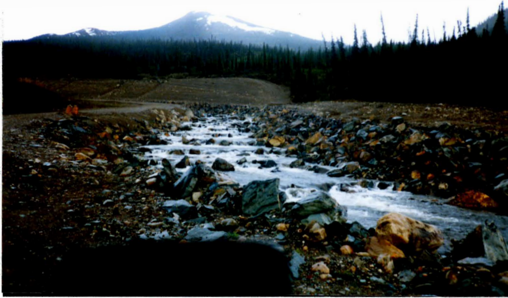
Photo 7 - Rose Creek diversion. Rip rapped section with heavier rap rapped velocity checks. This channel is in reasonable condition. Some of the large rip rap has moved. They should be moved back to original position.
