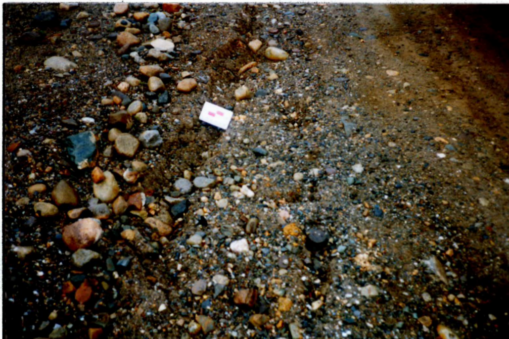
Photo 12 - A second crack with vertical displacement on the Rose Creek diversion dyke. This slide must be stabilized. If a major failure occurred Rose Creek could flow into the tailings pond.
