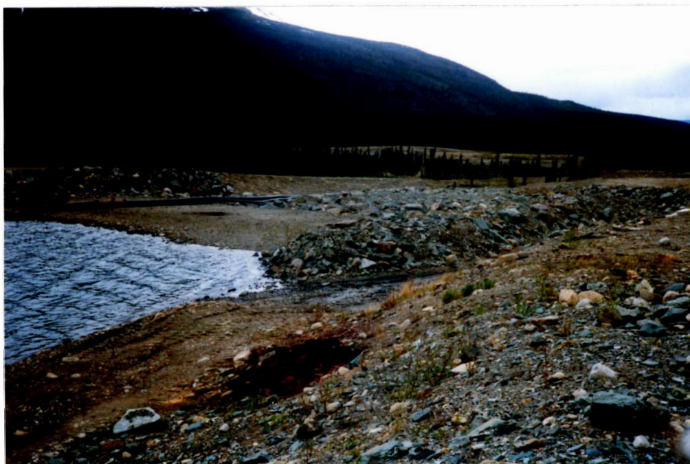
Photo 4 - Pipe siphon carrying water from lower pond over spillway location. North end Cross Valley dam.
