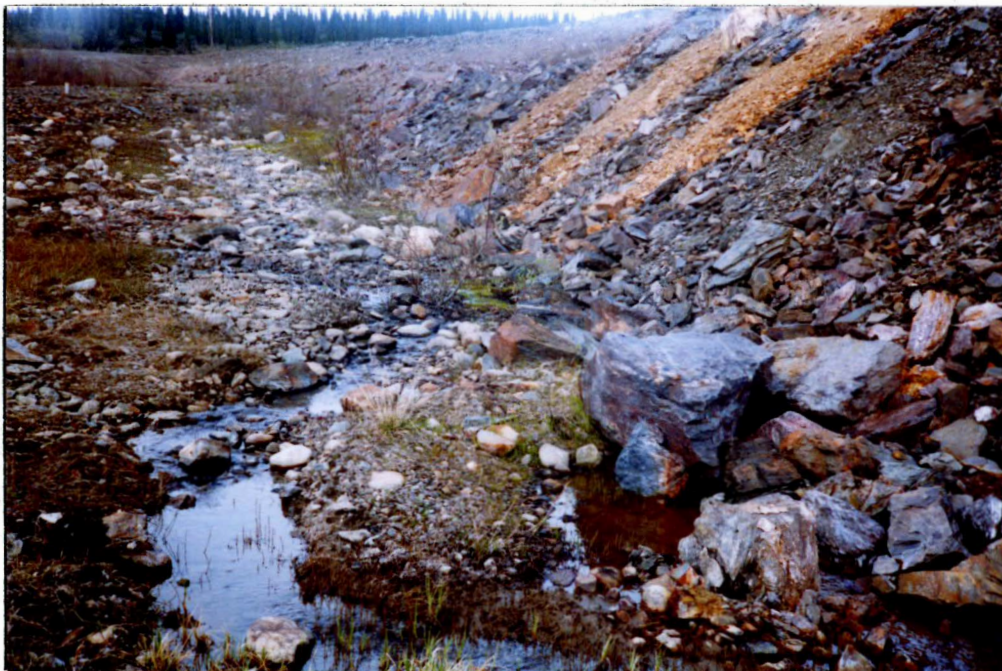
Photo 18 - Seepage at the toe of the berm below the fresh water dam. Several weeks prior to this inspection artesian pressures were monitored in a piezometer on the berm. The soil is spongy. The stability of this dam must be evaluated. It appears to have low stability.
