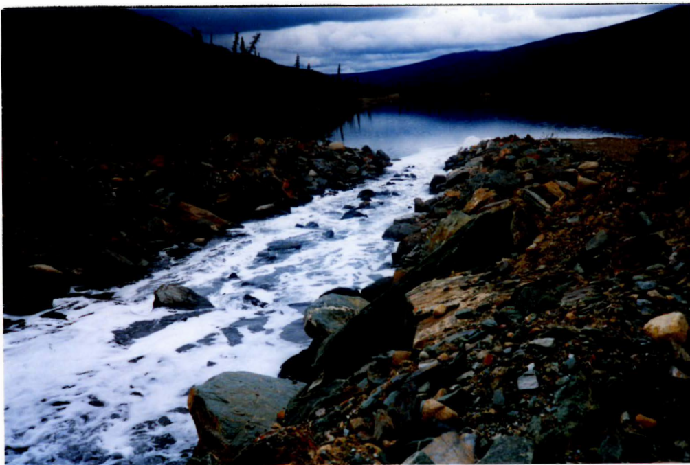
Photo 3 - Overflow rip rap spillway at the south end of the intermediate dam. This spillway is operating efficiently.
