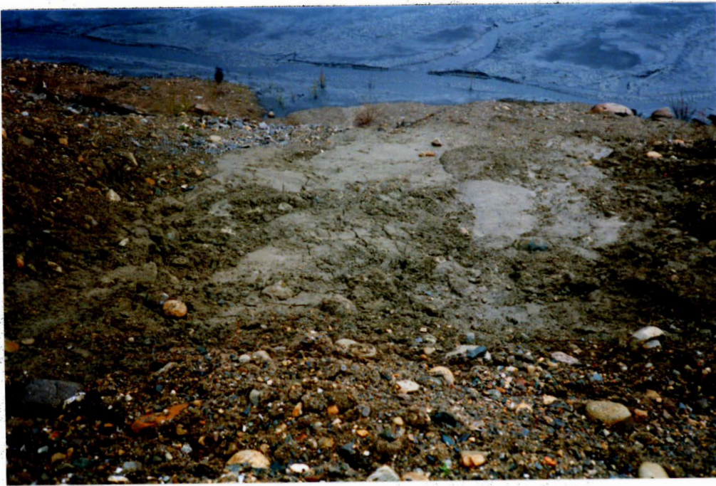
Photo.13 - Seepage and piping through Rose Creek dyke slope. This must be stabilized and controlled. This is occurring at several locations along the slope below the Rose Creek diversion.
