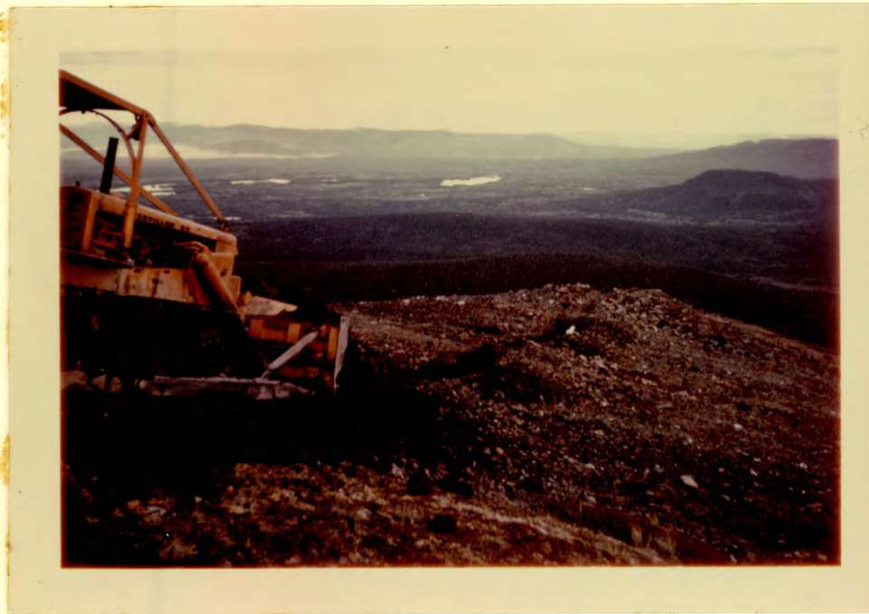
Start of trenches on North lead-zinc-silver showing with view of E-W lineament (valley in background).
