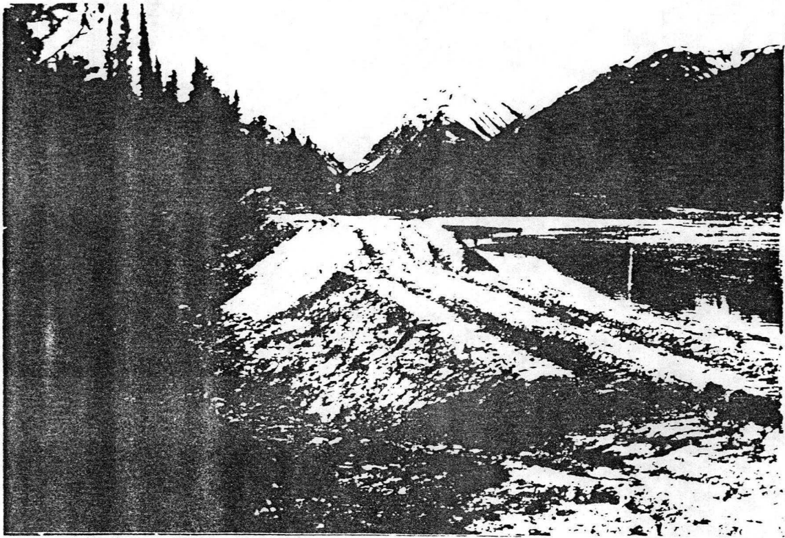
Photo 3: Dyke No. 3 - looking south. Current construction procedure involves pushing and spreading of the fill material (comprising powdery silt) with dozer.
