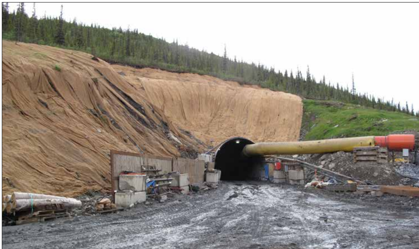
Portal into Bellekeno mine at Hecla Mining Company's recently acquired Keno Hill silver district.
