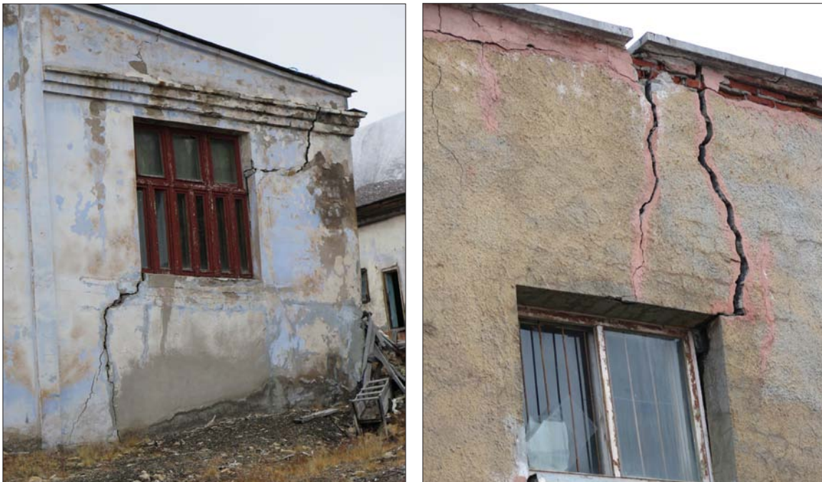
Figure F3. Examples of unmaintained buildings in Pyramiden, Svalbard, displaying cracks and uneven settlement in response to permafrost thaw.
