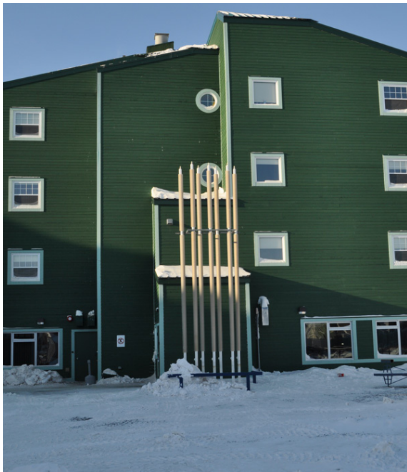
Figure F16. Example of thermosyphons, a foundation system that requires a significant amount of expertise to design, install, maintain and monitor (CSA, 2014).
