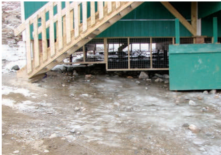
Figure F18. Example of water ponding around a foundation built on permafrost (Government of Nunavut, 2013). Water ponding can have a negative impact on permafrost thermal regimes.
