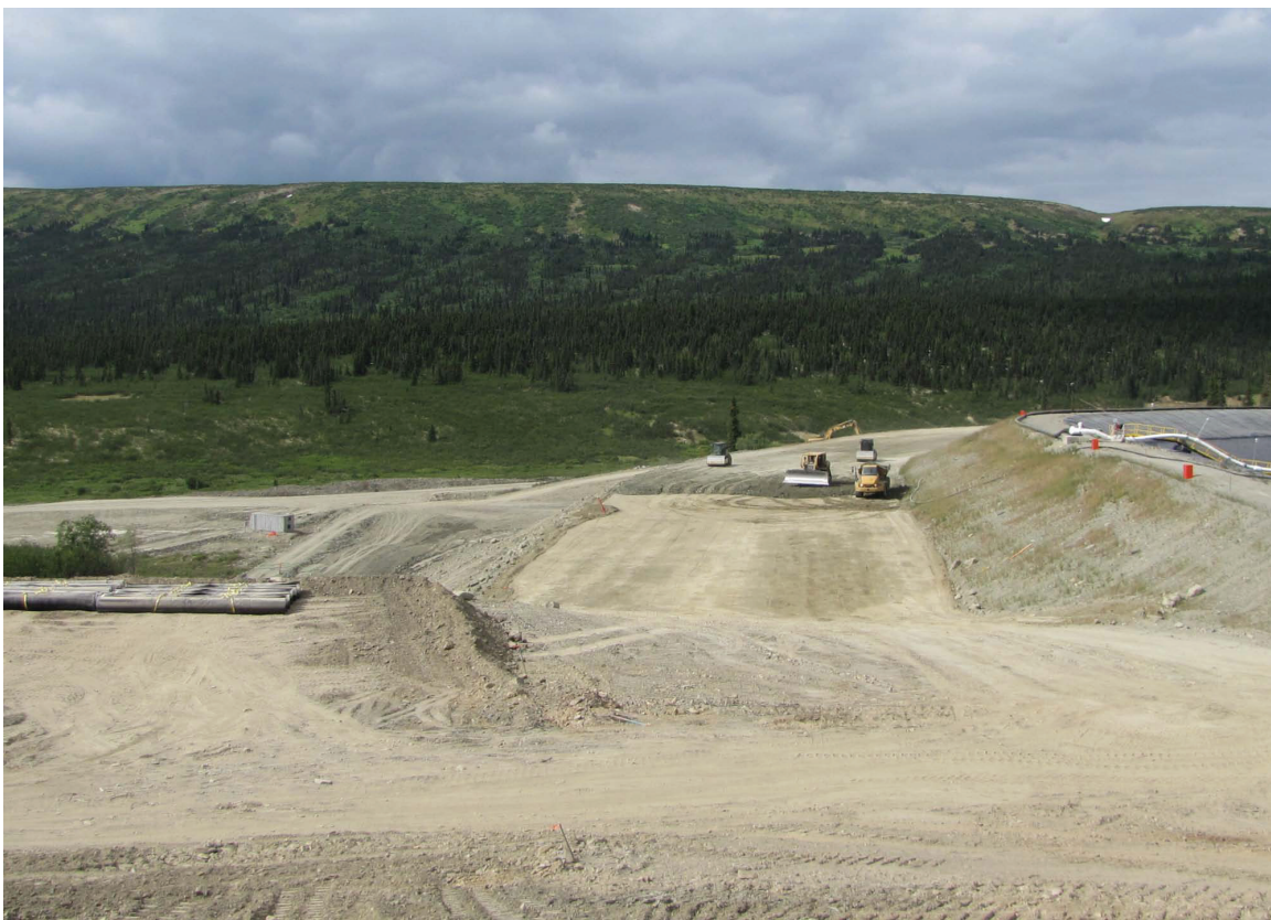
Figure 3. Equipment placing and compacting material on the tailings dam lift. Photo - courtesy of Glenn Ford, Water Resources.
