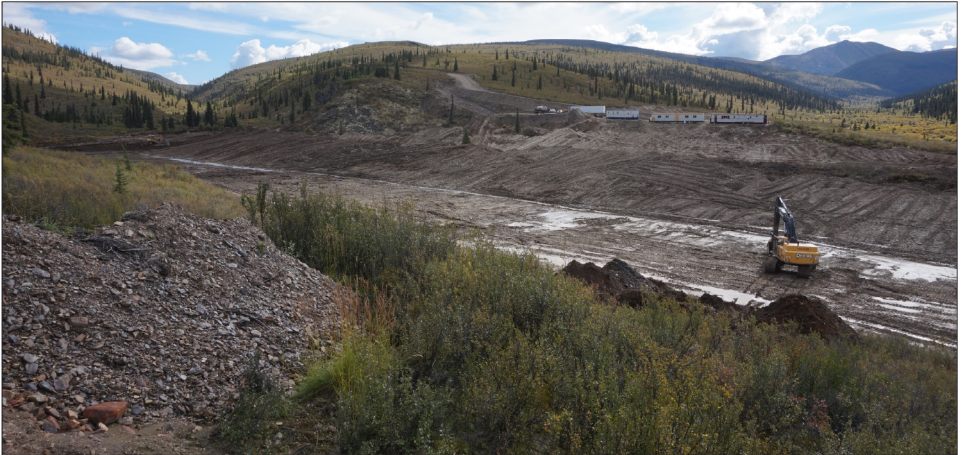
Figure 18. A view to the southwest of Schmidt Mining's operation on a tributary to Big Creek. Big Creek is the valley visible on the right side of the photograph looking toward West Ridge.
