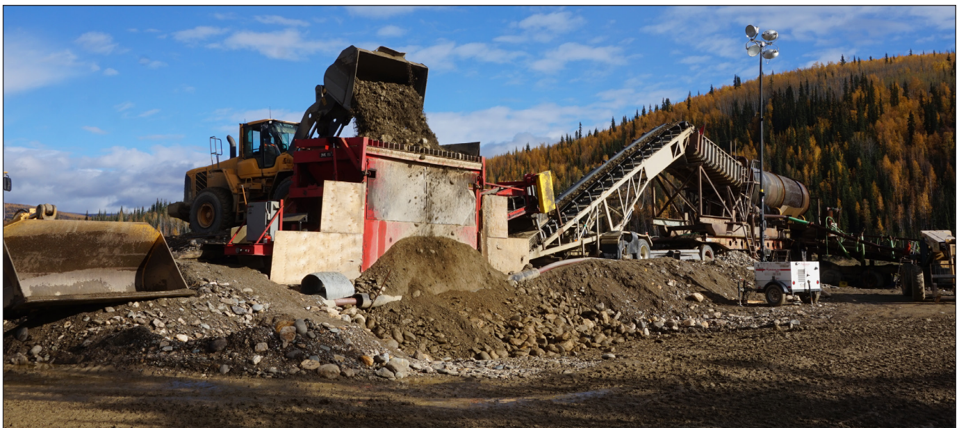
Figure 17. Storm Structures wash plant on Barlow Creek.
