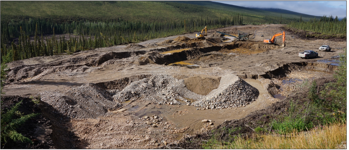
Figure 14. M2 Gold's operation on the 60 Mile River bench in 2016. A 50 m-wide cut was processed along the rim of the bench using two excavators and a mobile plant.
