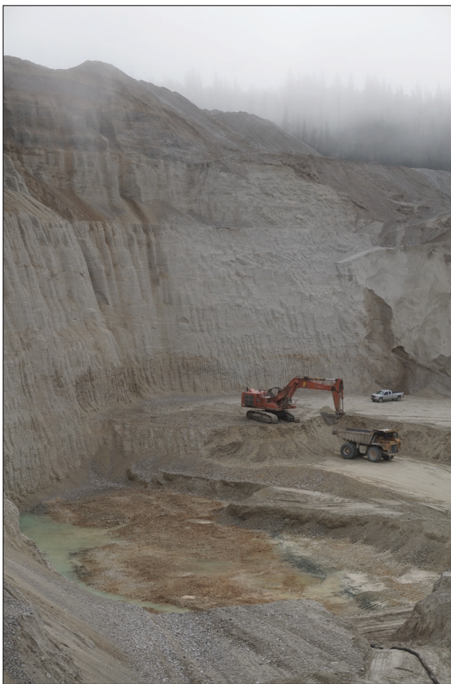
Figure 8. A view of the Lovett Hill cut in 2019 showing the orange bedrock surface near the excavator. Undocumented underground old-timer workings from 1917 (based on a preserved newspaper) were discovered in the vicinity of the cut.
