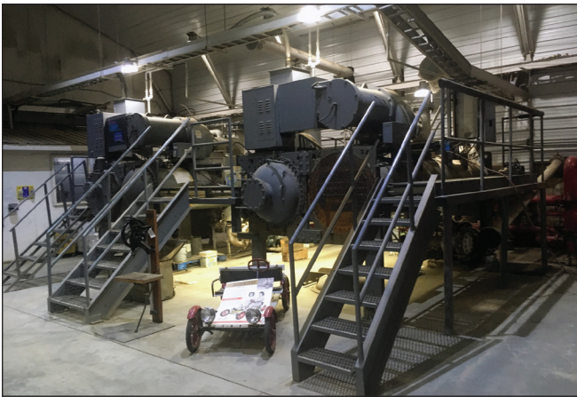
Figure 16. Two binary-system power plants generate 0.4 MW of electricity at the Chena geothermal plant.
