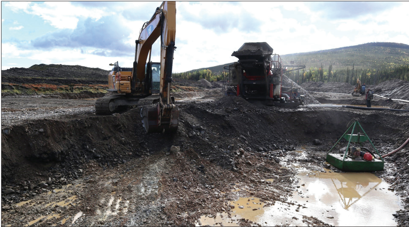
Figure 12. A view of M2 Gold Mines' plant on the Sixtymile River. Their mobile trommel plant reduces costs associated with hauling pay gravel.
