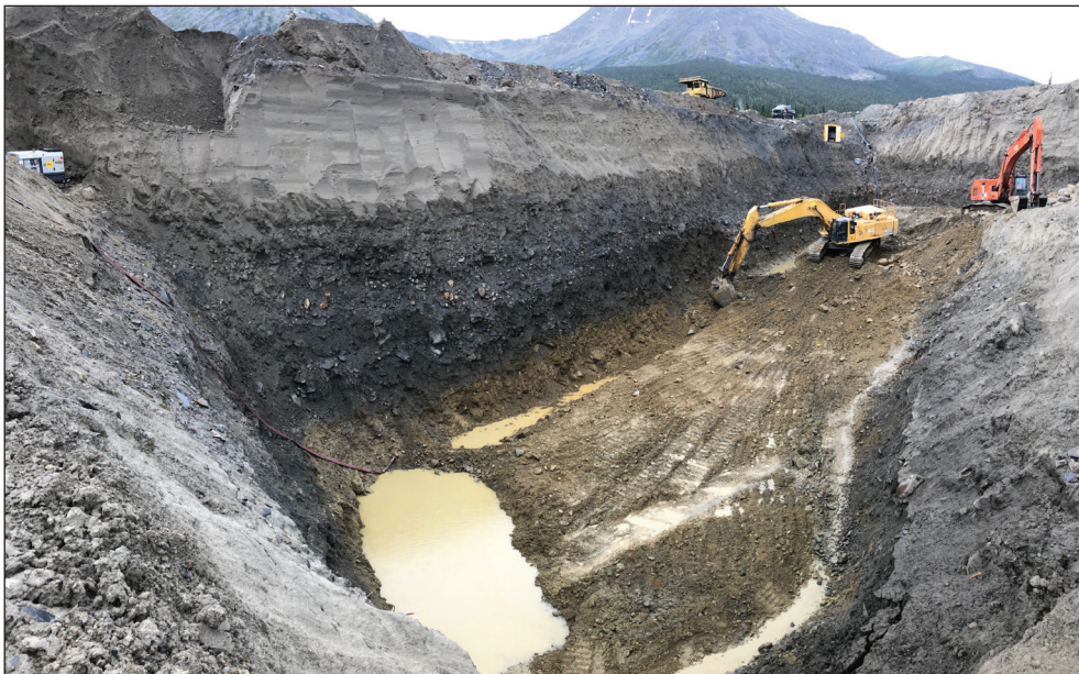
Figure 19. Dulac Mining's cut on Granite Creek in 2020. The oxidized till exposed at the base of the cut represents the top of the pay unit and was deposited by a pre-last glacial advance of a local alpine glacier.
