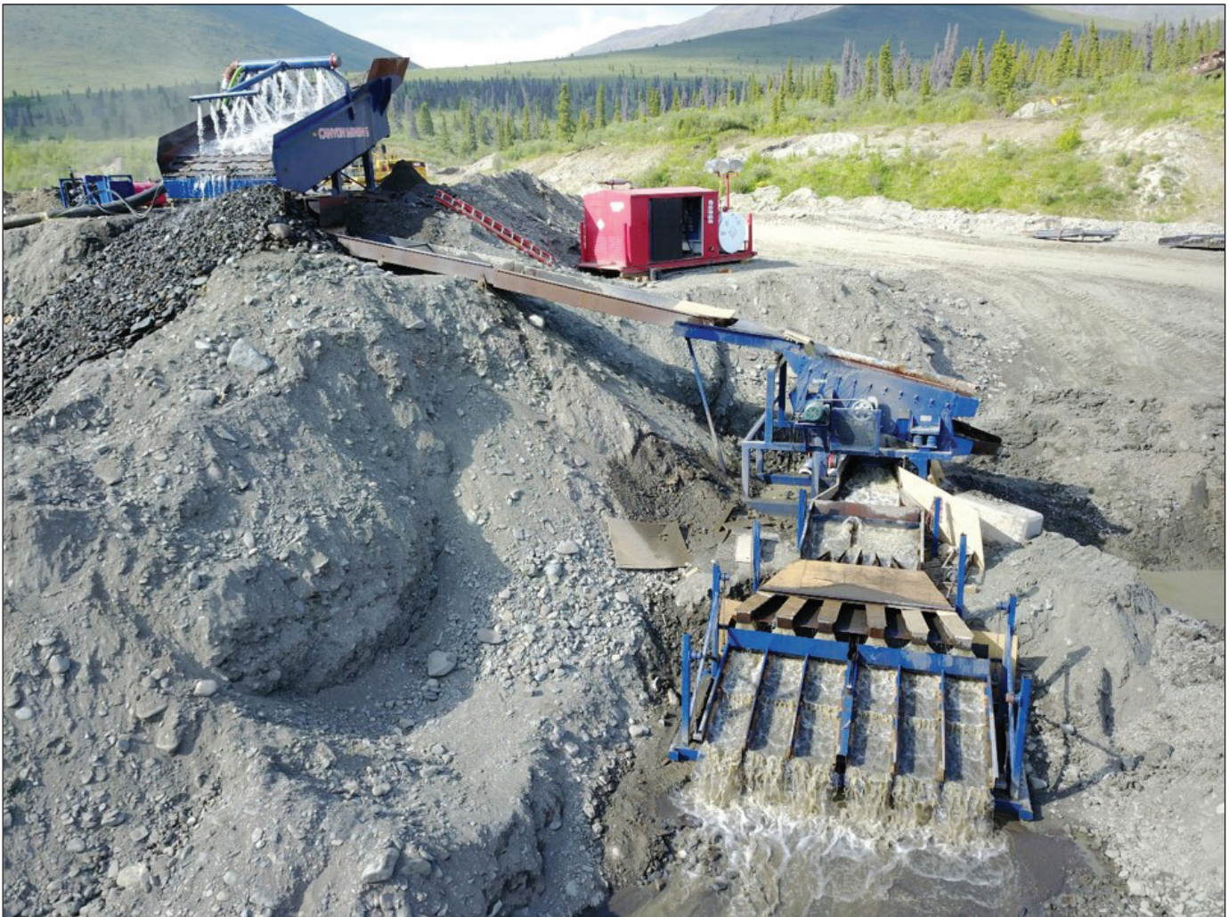
Figure 22. Canyon Mining Limited's wash plant and sluicing configuration on Fourth of July Creek.
